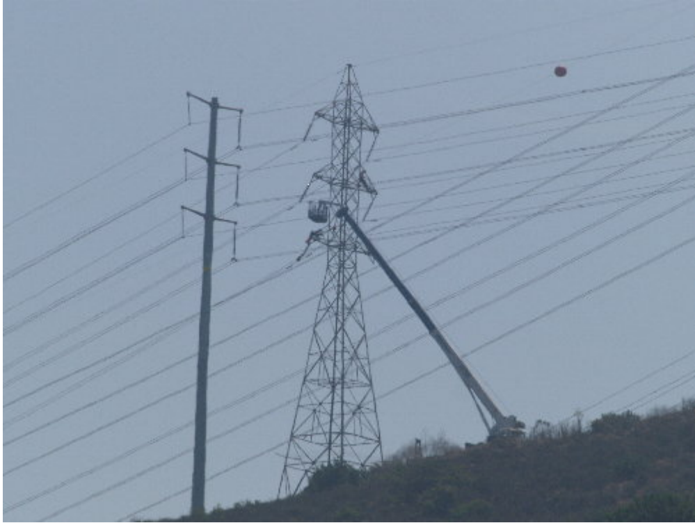
Figure 1 – The Wilson crew worked in the Sweetwater area dropping conductor from towers that will either be modified or replaced by steel poles.
