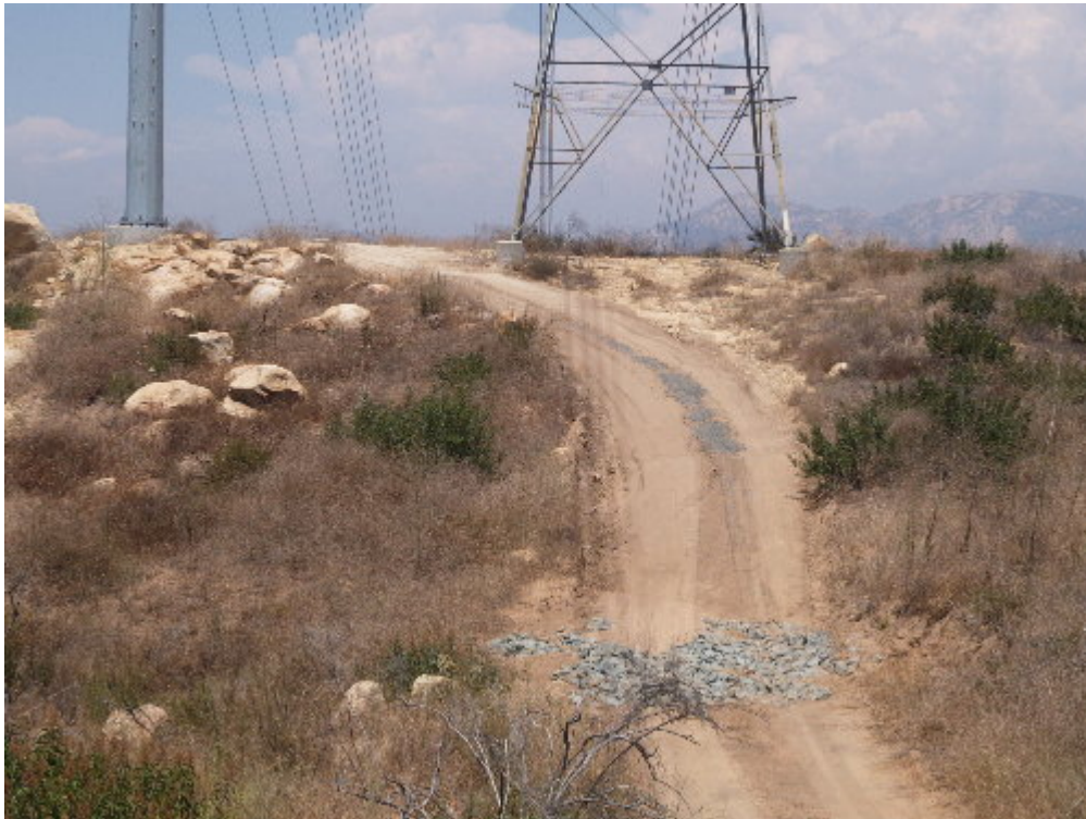
Figure 6 – A minor concrete spill near Tower Site 16. Note that the dip at the lower spot in the road is rock placed to control erosion, not concrete.
