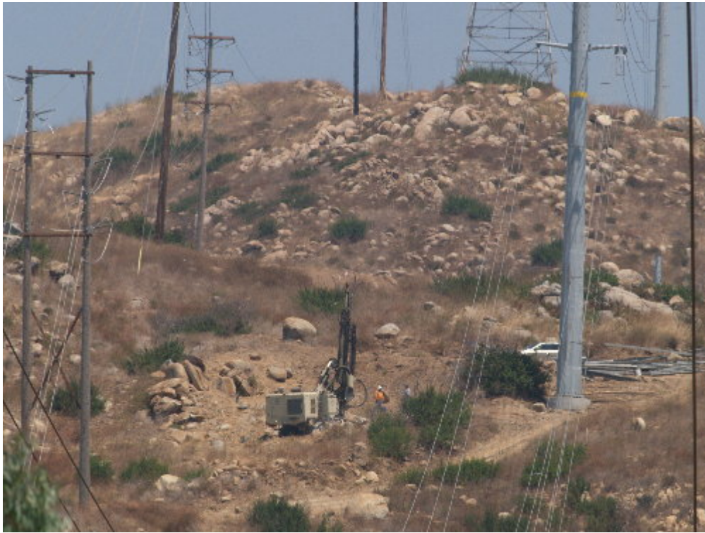
Figure 3 – A drilling subcontractor worked east of Hillsdale Street to test for rock with a small-diameter drill head.
