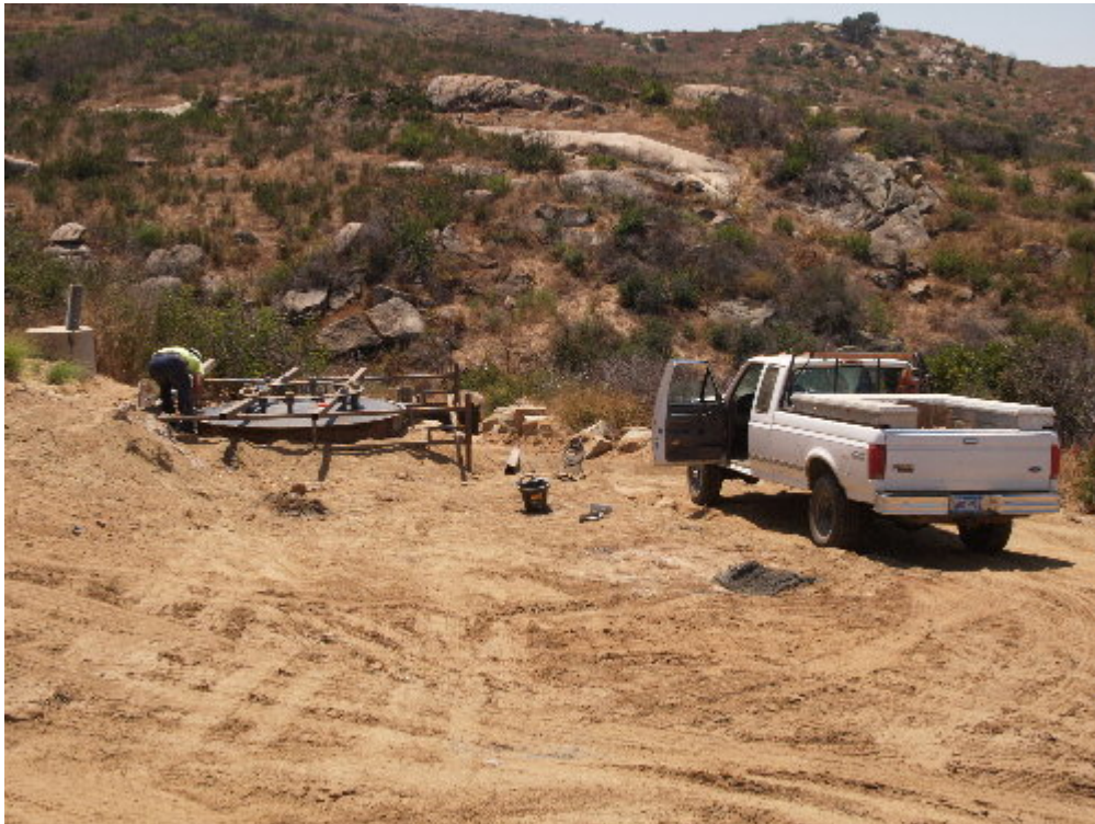
Figure 4 – Tri-State Drilling crews poured the foundations for new steel poles. An inspector from Testing Engineers was on-site.
