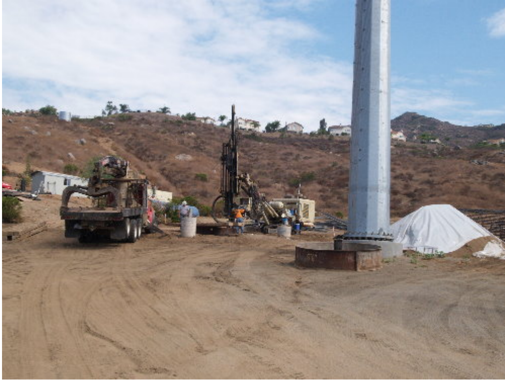
Figure 1 – Edick and Watt worked east of Hillsdale Street to test for rock with a small-diameter drill head.
