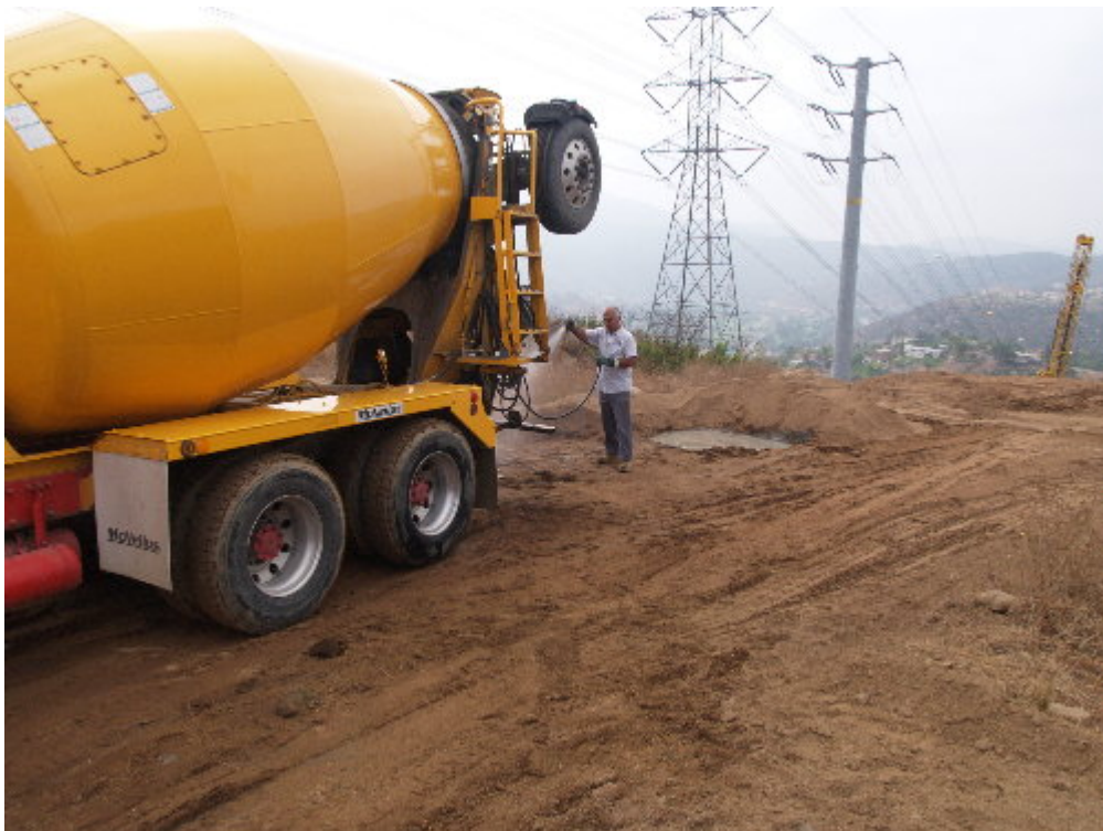
Figure 4 – The concrete truck drivers washed out in the approved area that will be cleaned out after the pour.
