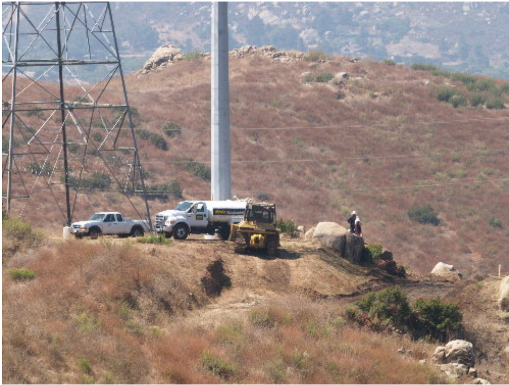
Figure 5 – The Tri-State Drilling crew worked to prepare the pad and access to Tower Site 24 for drilling.
