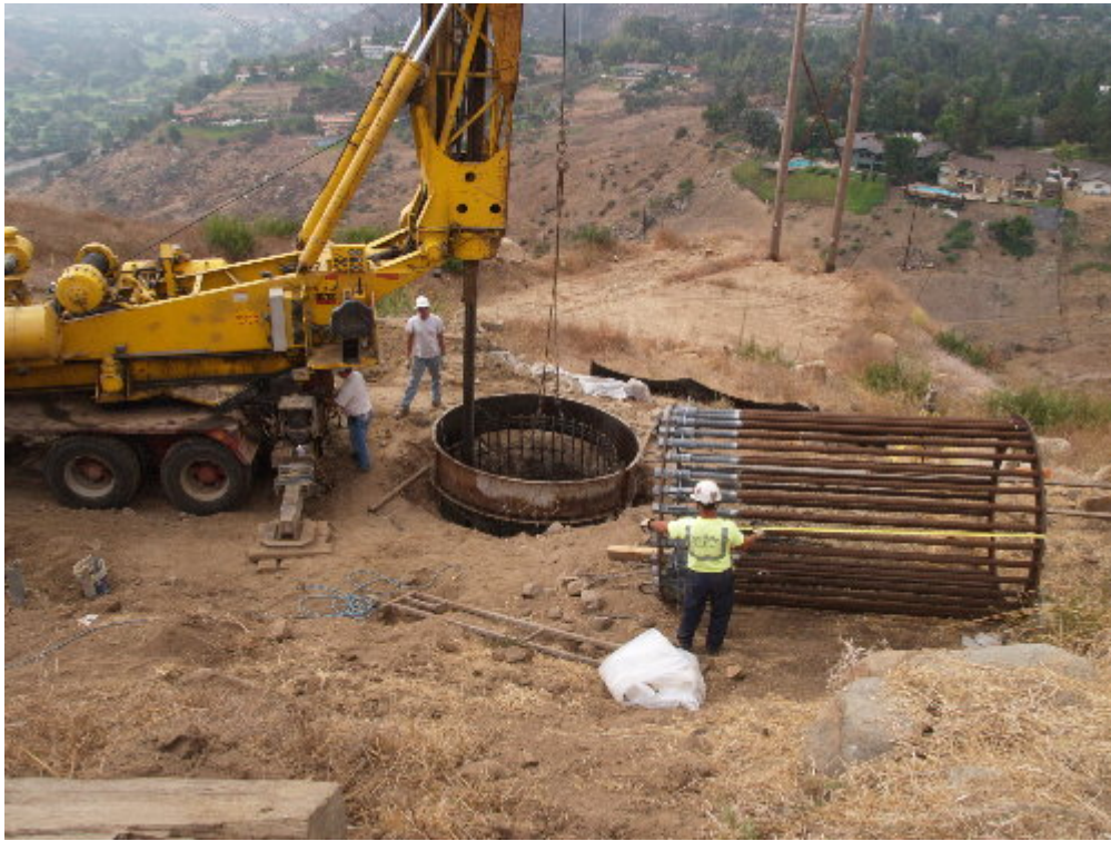
Figure 3 – The Tri-State Drilling worked to support the rebar cage during the concrete pour.
