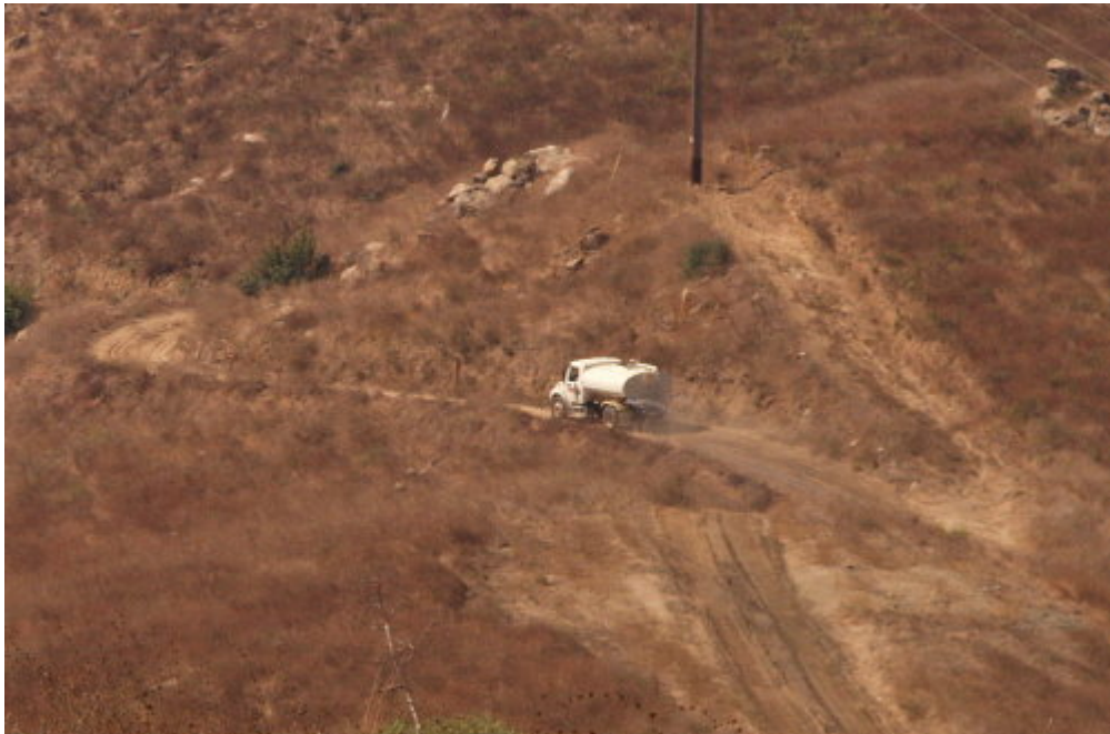
Figure 6 – The Tri-State water truck controlled fugitive dust on the access to Tower Site 26 during spoil removal.
