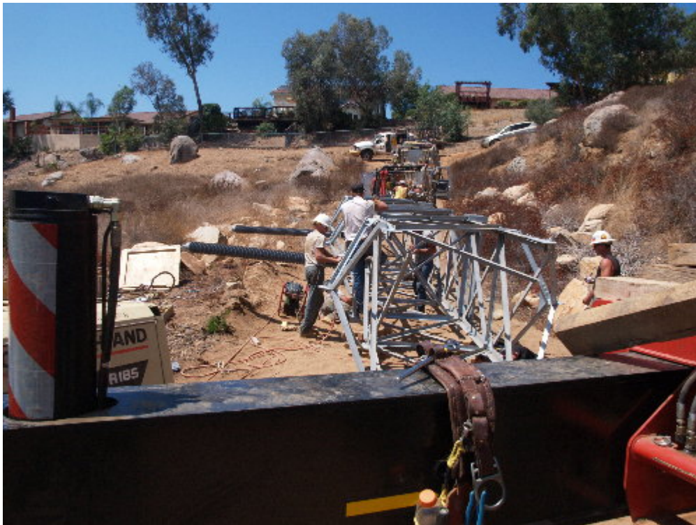
Figure 2 – Wilson crews worked to modify the top of the tower before reattaching it to the lattice structure.
