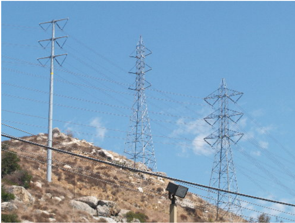
Figure 3 – The center structure has been modified by the Wilson crew.
