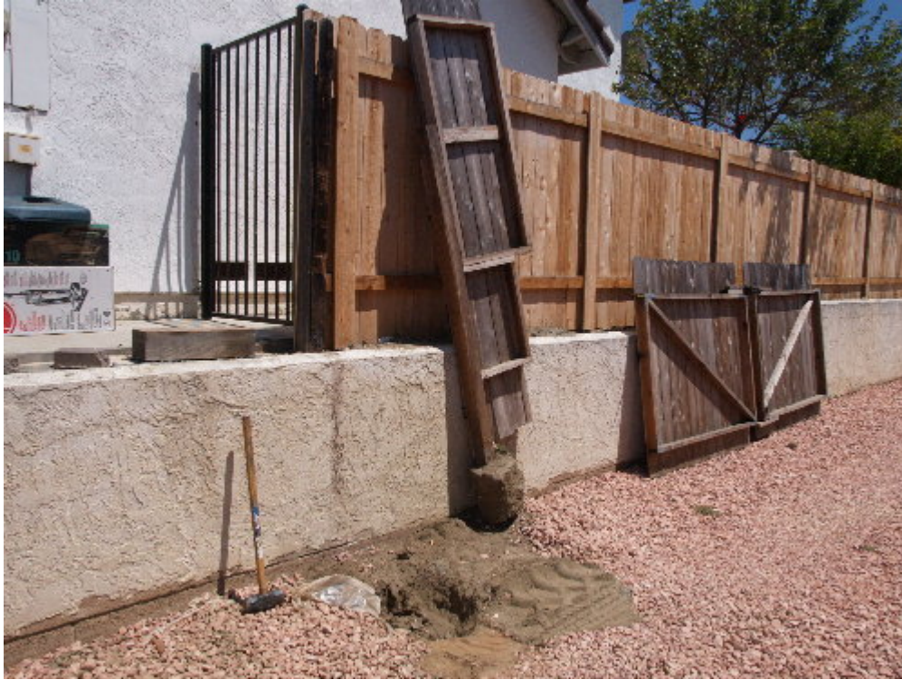
Figure 1 – The property owner gate was removed to allow access for the crane off Wind River Drive.
