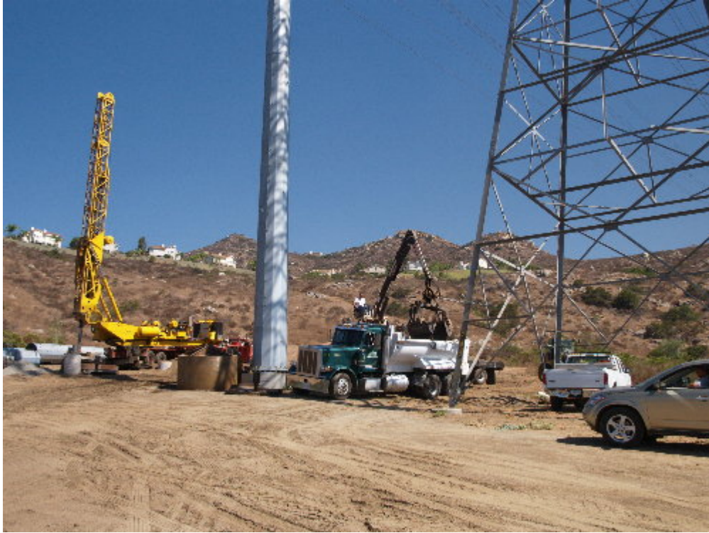
Figure 1 – The Tri-State drilling crew worked to removed excess spoils from the Tower 9 site during the site visit.
