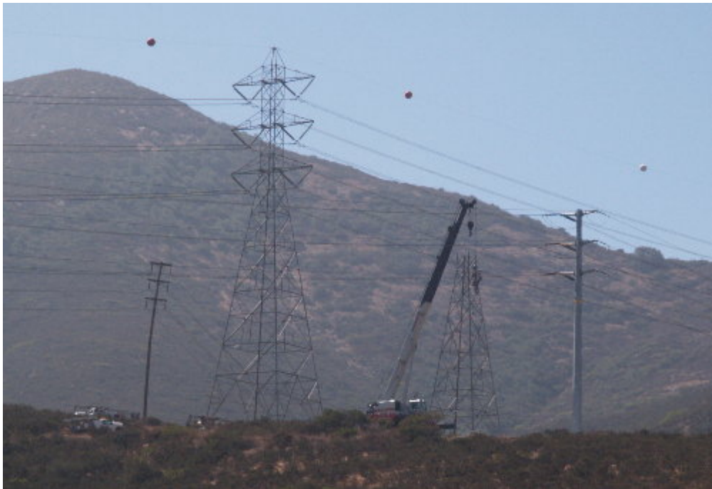
Figure 4 – The Wilson tower modification crew worked west of Millar Ranch Road during the site visit.
