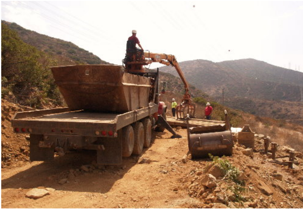
Figure 3 – The Tri-State drilling crew set timber mats on the excavation in preparation for blasting.
