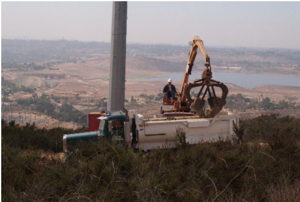
Figure 2 – The excess spoils were removed following the excavation of the foundation above Sweetwater.
