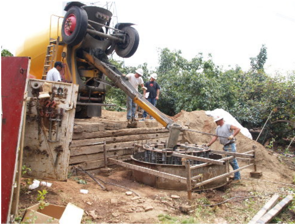
Figure 1 – The Tri-State drilling crew placed concrete in the excavation off Singing Vista.
