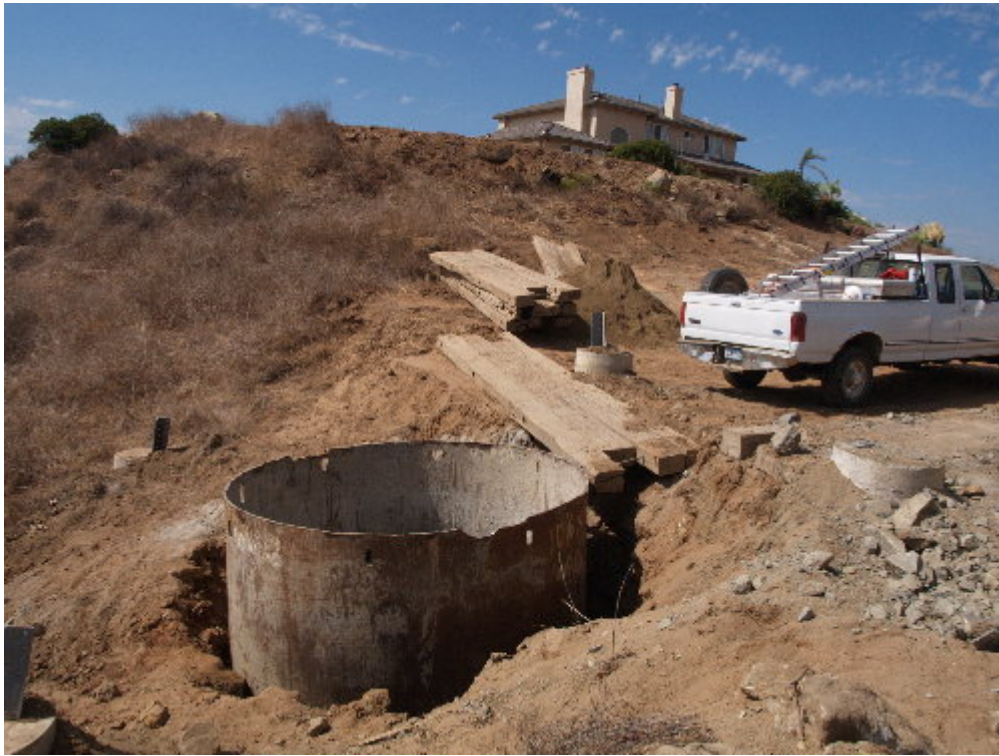
Figure 3 – The Tri-State drilling crew stopped drilling at Site 32 and will bring the blasting contractor back to address additional rock.
