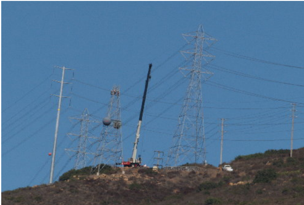
Figure 4 – The Wilson tower modification crew worked at Tower 62 during the site visit.
