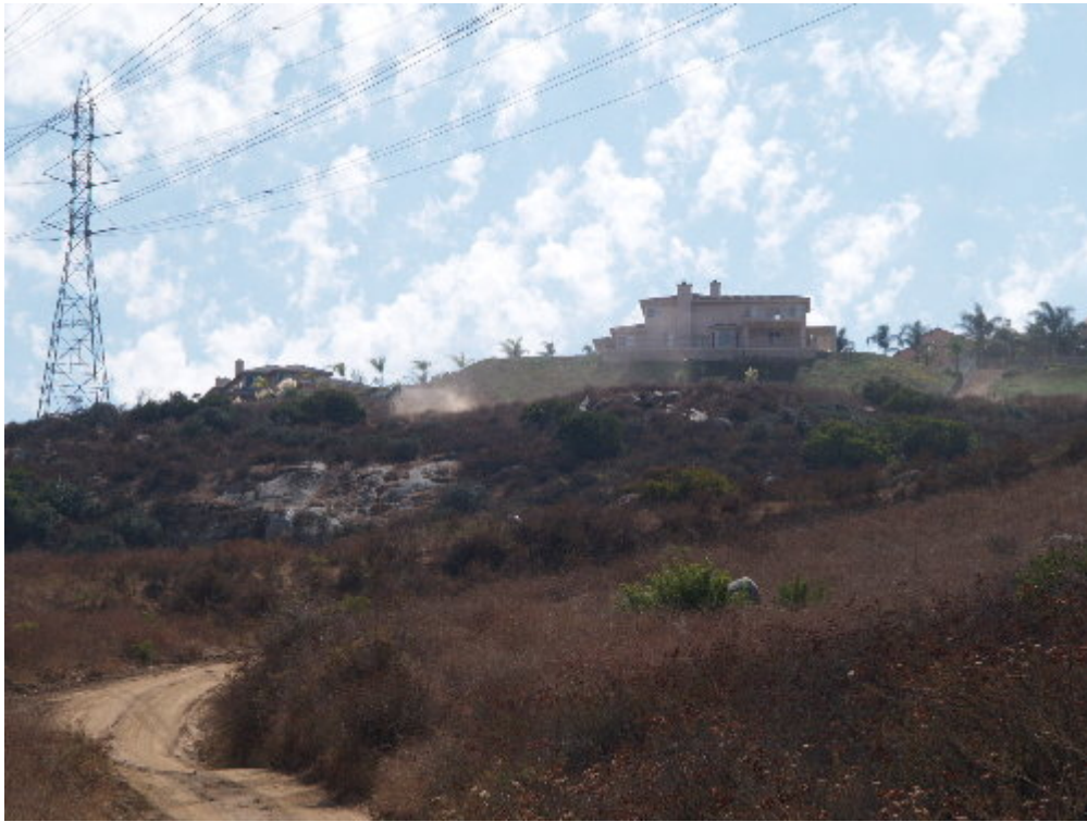
Figure 5 – Fugitive dust was observed during the hauling of excess spoils from Pole Site 32.
