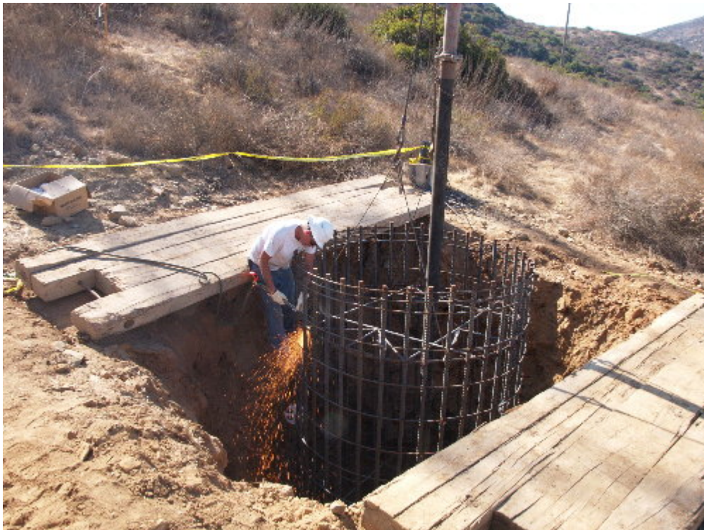
Figure 2 – The cross supports were removed from the rebar cage once it was lifted into place.
