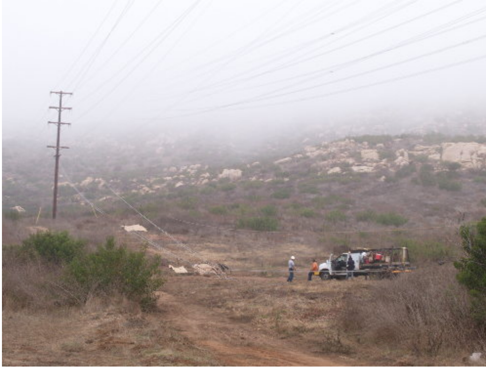
Figure 1 – The reel trucks were staged in the approved stringing site east of La Cresta during the sagging operation.
