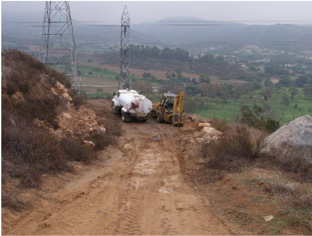
Figure 3 – A crew worked to repair the slopes at Tower Site 39 during the site visit.
