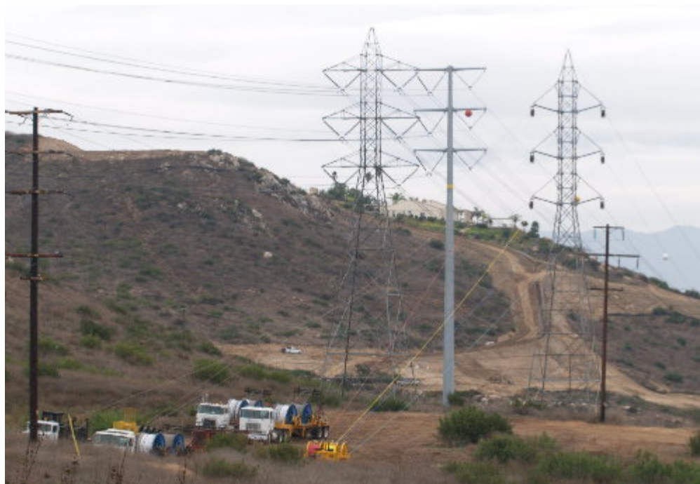
Figure 1 – The reel trucks were staged in the approved stringing site east of La Cresta in preparation for pulling conductor.
