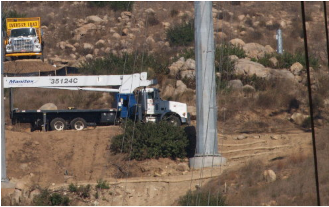
Figure 3 – The fiber rolls below the pad off Camino Monte Sombra need maintenance and improvement. Note the gaps under the fiber rolls.
