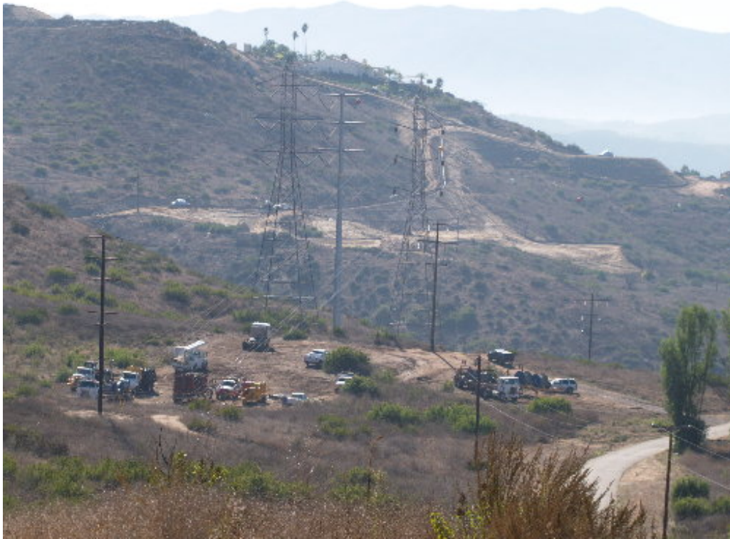
Figure 1 – The reel trucks were staged in the approved stringing site east of La Cresta during the sagging of the strung conductor.
