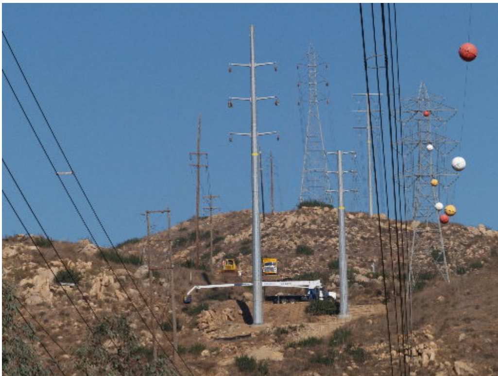
Figure 2 – A second crew was set up off Camino Monte Sombra during the stringing and sagging operation.
