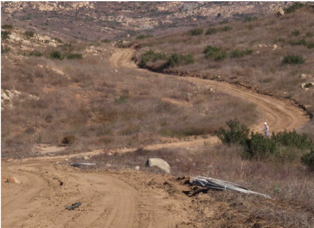
Figure 3 – The damaged conductor was cut into smaller sections and rolled by hand since the reel truck was not available. Note the conductor going through the vegetation up the left side of the photograph.
