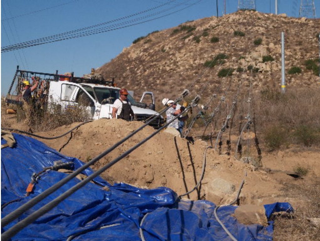
Figure 1 – A Wilson crew was set up off Camino Monte Sombra during the stringing and sagging operation.
