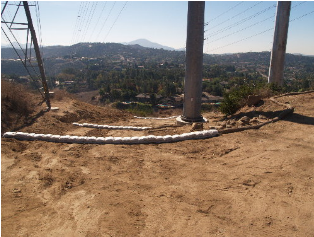
Figure 2 – The BMPs were repaired and augmented below the stringing operation at Tower 25.
