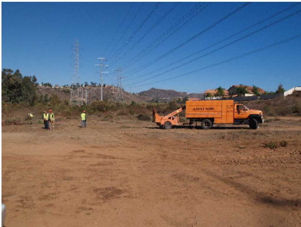
Figure 4 – The clearing crew worked on the edges of the approved laydown area on the east side of the Herrick Center.
