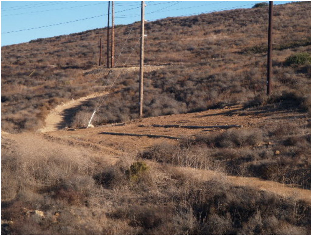
Figure 5 – The fiber rolls and water bars on the old stringing site near the Miguel Substation have been increased and improved.
