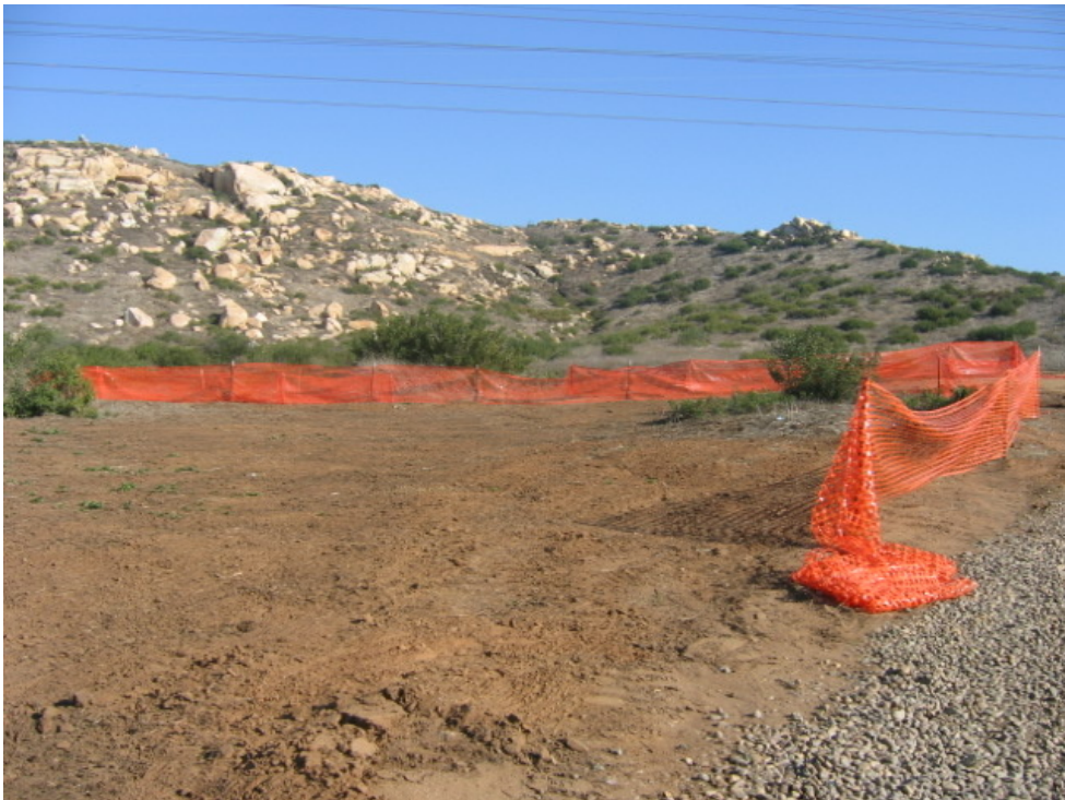
Figure 2 – Wilson crews performed grading for a stringing site at Miguel and installed BMPs.
