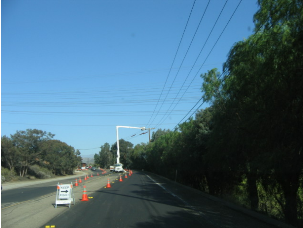
Figure 1 – A boom truck was used to protect the 12 kV lines during stringing near the Cottonwood Golf Course.
