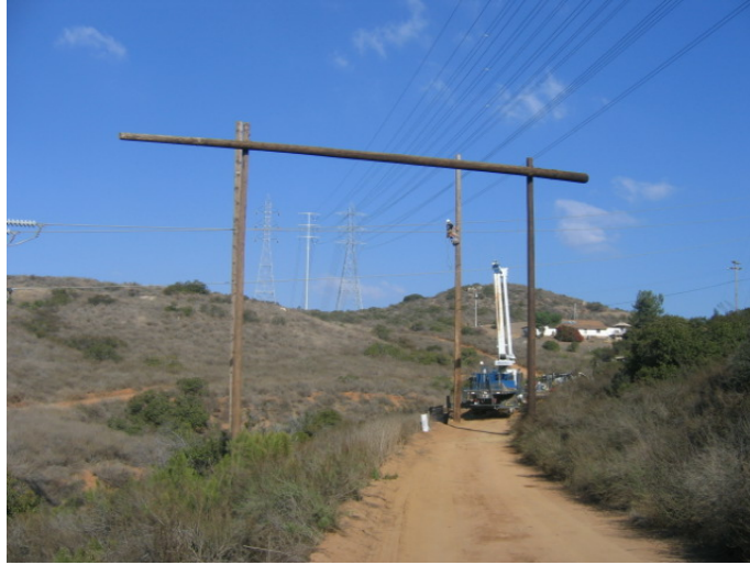
Figure 1 – Construction of guard structure over active power line near Steel Canyon High School.
