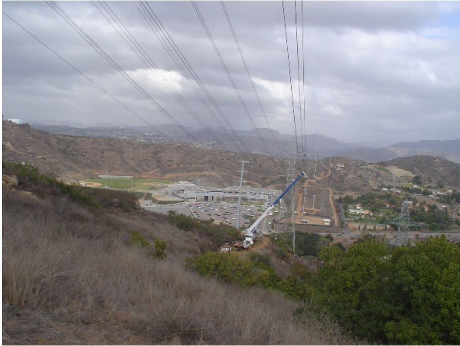
Figure 1 – Clipping in of the conductor near Tower 49. Steel Canyon High School is in the distance.
