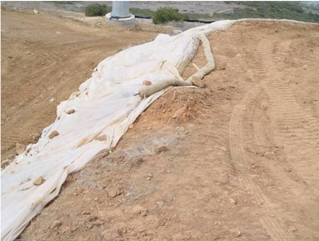
Figure 2 – Plastic sheeting needs to be keyed into top of slope and straw wattles on slope need to be properly installed.
