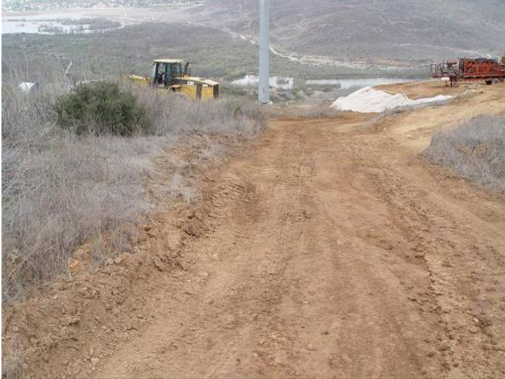
Figure 1 – Location of off right-of-way incident near Tower 132 due to slippery road conditions. Area impacted was approx. 4 by 20 feet.
