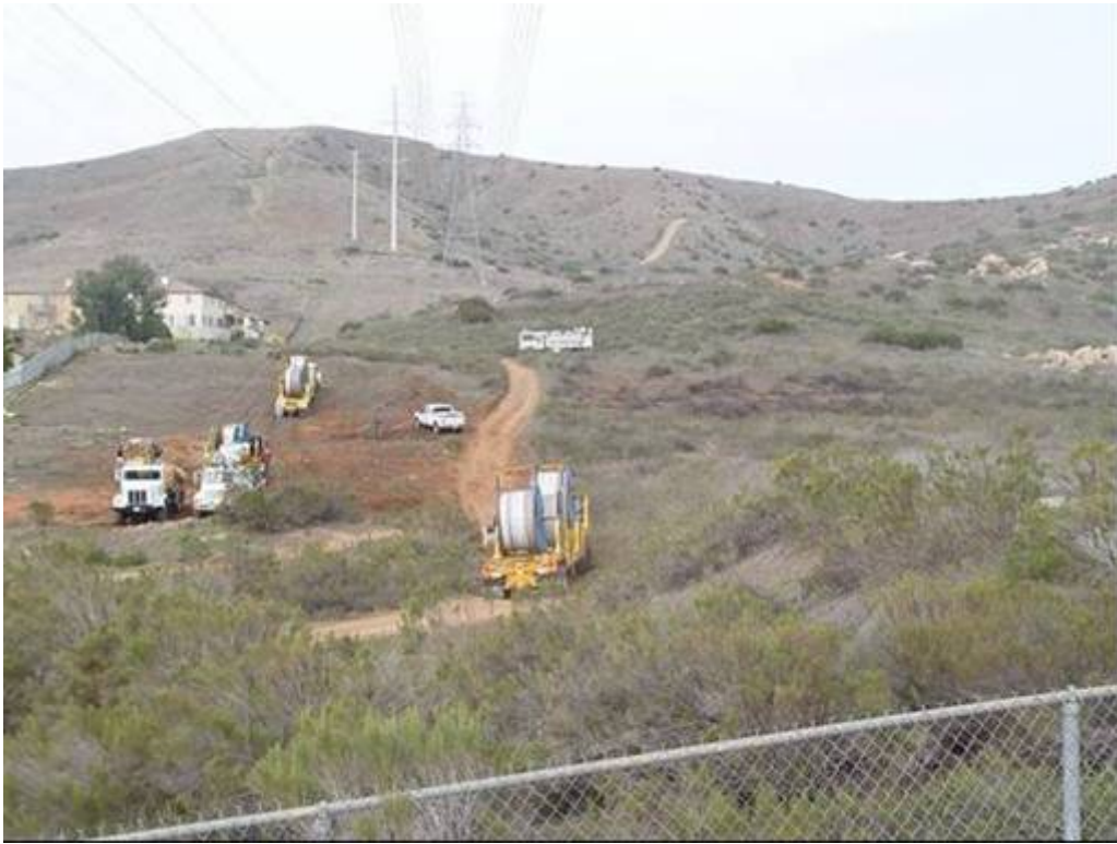
Figure 3 – The reel truck in the foreground is the truck and exact turn where incident occurred. The truck length and turning radius caused the issue on the tight access road.
