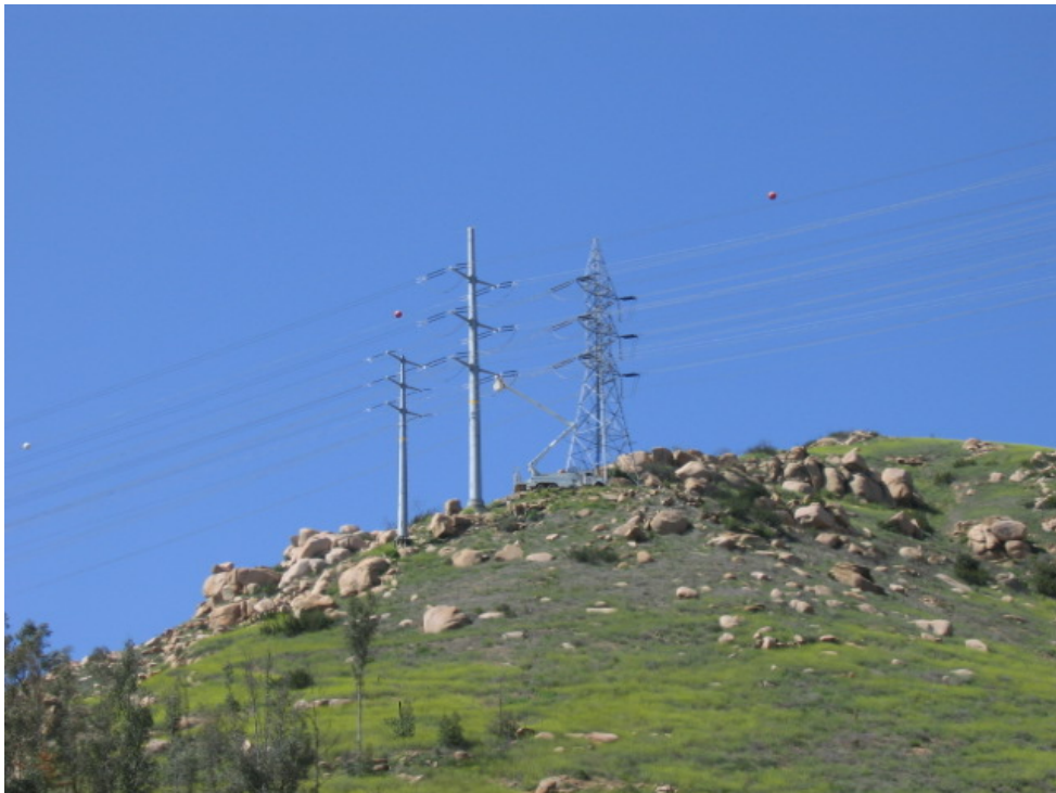
Figure 2 – PAR crews completed installing the last section of wire installation on the Fanita to Los Coches segment.
