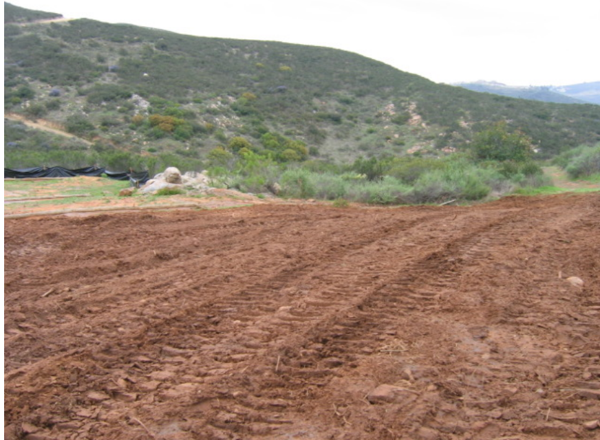
Figure 1 – A snub site used by Wilson crews near Structure 52 has been recompacted and erosion control measures have been installed.
