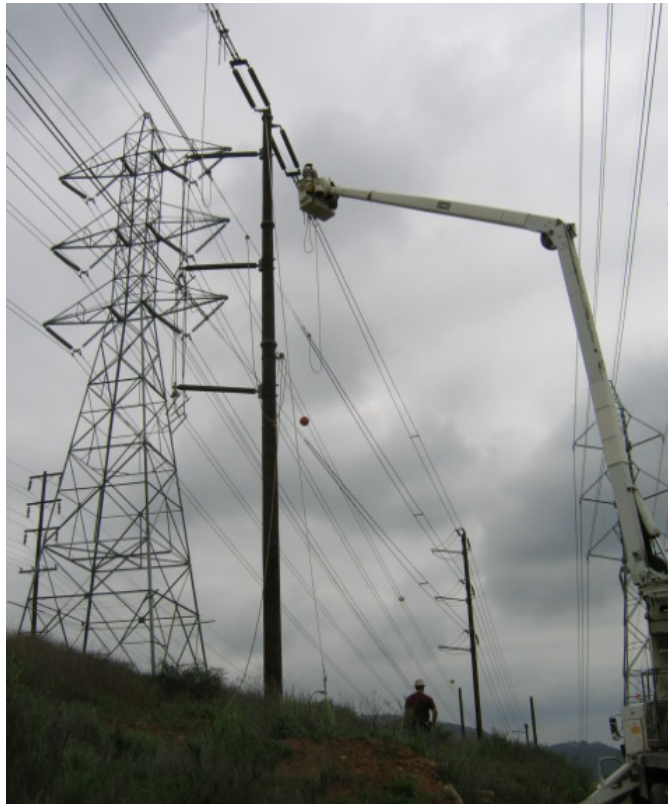
Figure 2 – Sturgeon crews working on the temporary 230 kV lines near Lake Jennings. The “put back” involves reconfiguring the wood poles to accommodate a double circuit of smaller kV lines.
