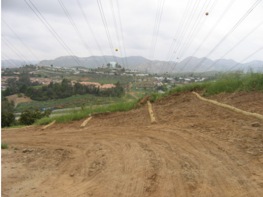
Figure 1 – A tower pad site used by Wilson crews near Highway 8 has been recompacted and erosion control measures have been installed.
