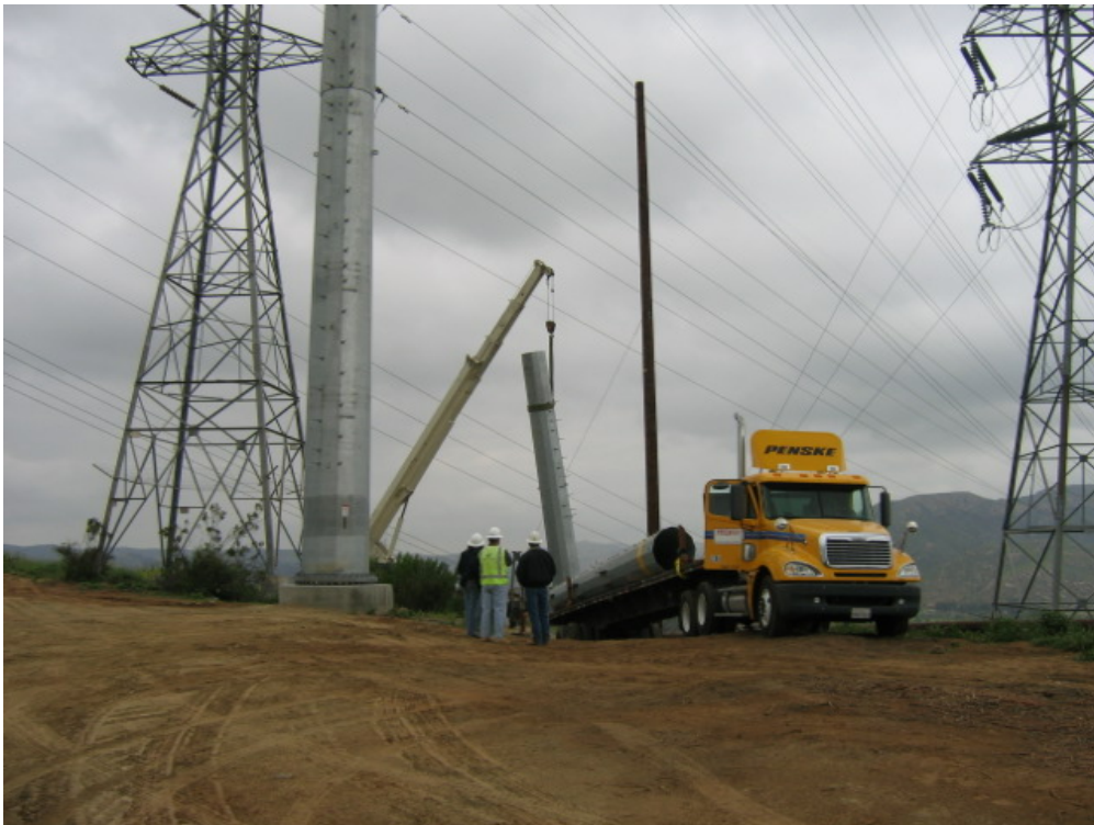
Figure 2 – Sturgeon crews working on the temporary 230 kV lines near Lake Jennings. The “put back” involves reconfiguring the wood poles to accommodate a double circuit of smaller kV lines.
