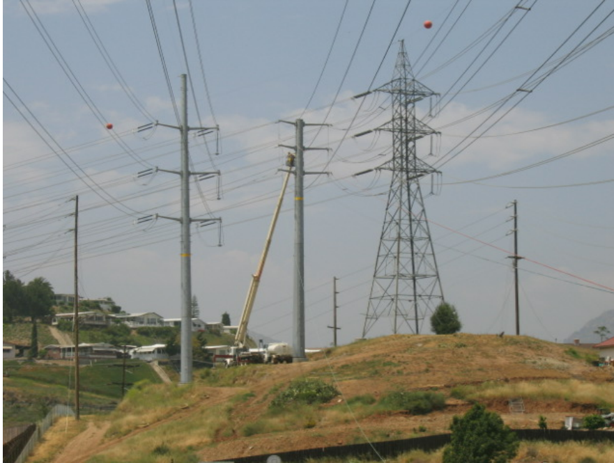
Figure 1 – Sturgeon crews working on the temporary 230 kV lines near Lake Jennings. The “put back” involves reconfiguring the wood poles to accommodate a double circuit of smaller kV lines.
