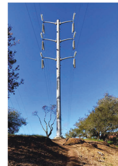
Tubular steel pole
