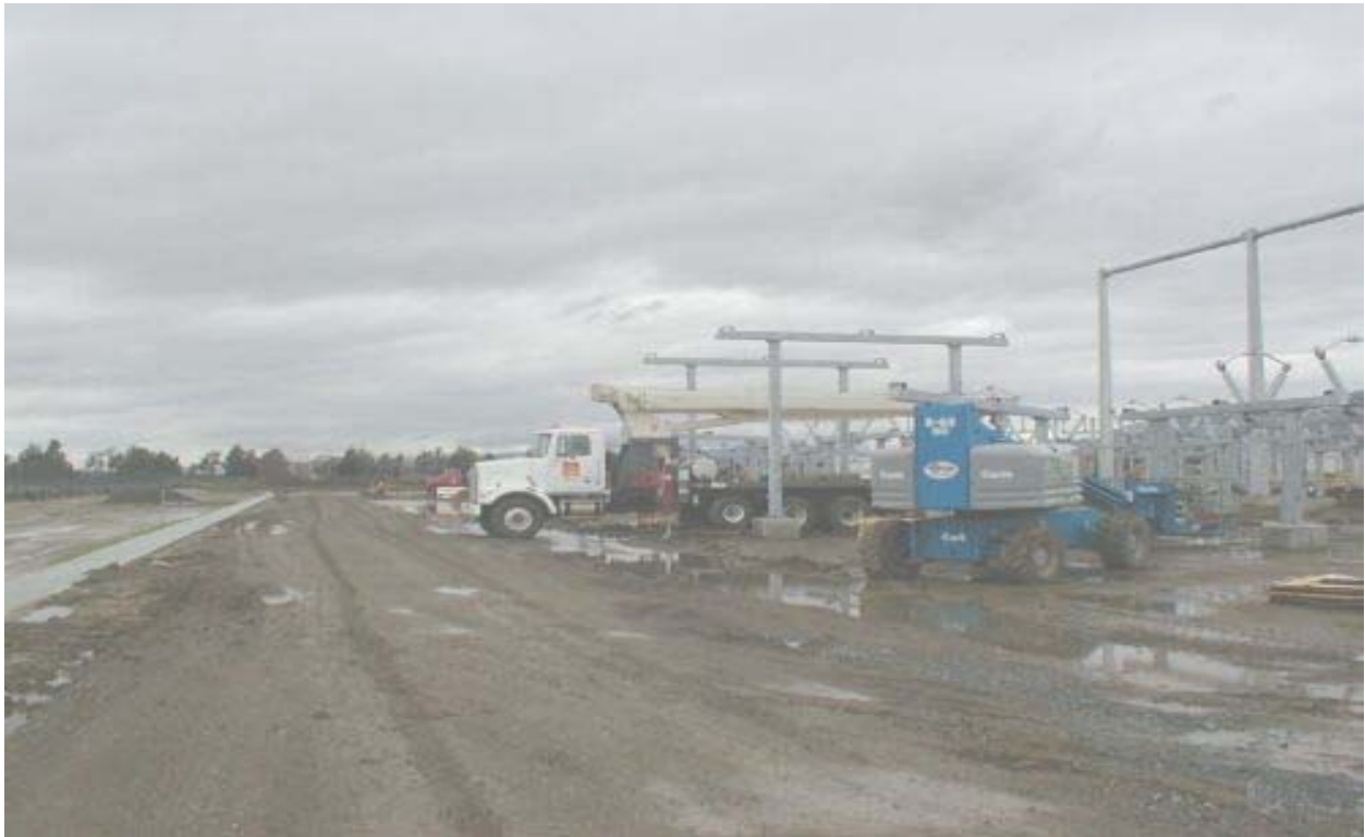
Figure 6 Los Esteros Substation – View of Drain Along West Side of Site January 10, 2003
