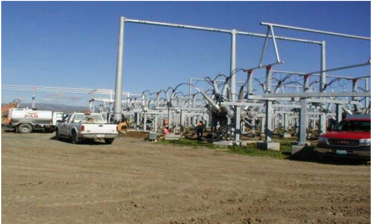
Figure 2 Los Esteros Substation March 26, 2003
