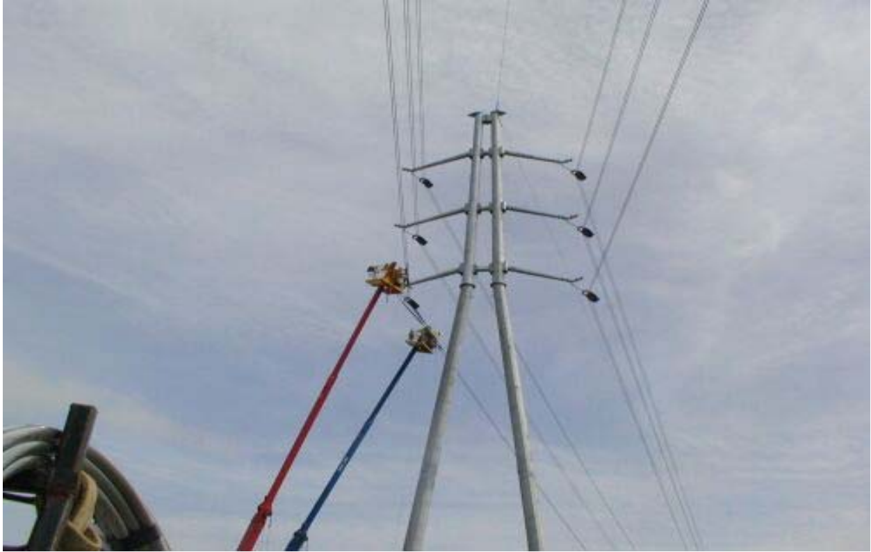
Figure 1 Pole Structure #5 March 26, 2003
