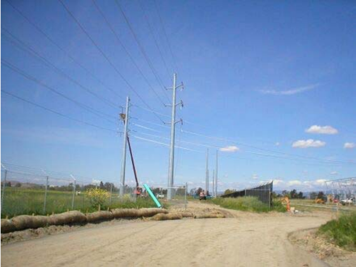
Figure 3 Cable Stringing in the Field West of the Los Esteros Substation April 5, 2003
