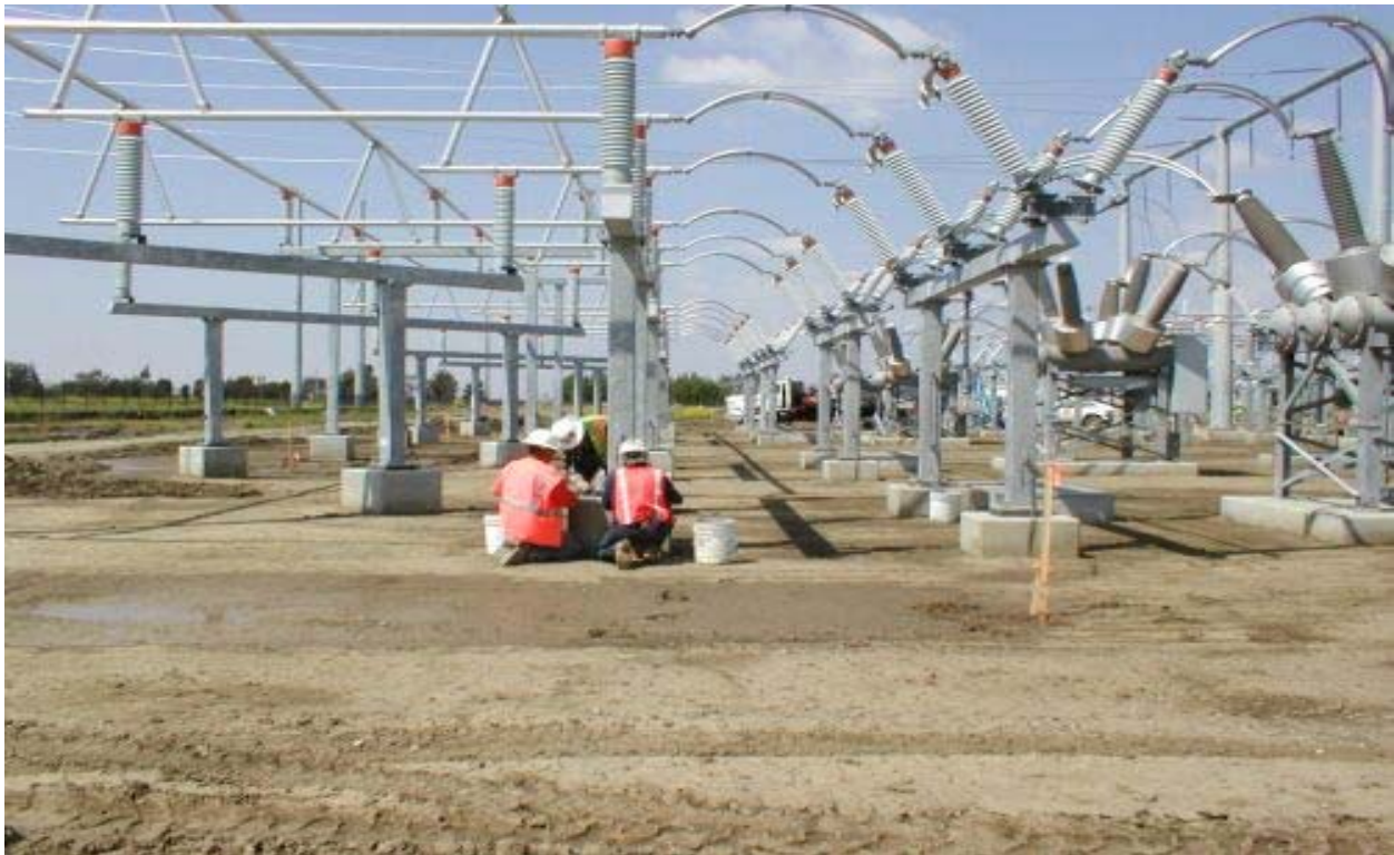
Figure 2 PAR Crews Grouting Between Steel Structures and Foundations at Los Esteros Substation April 18, 2003
