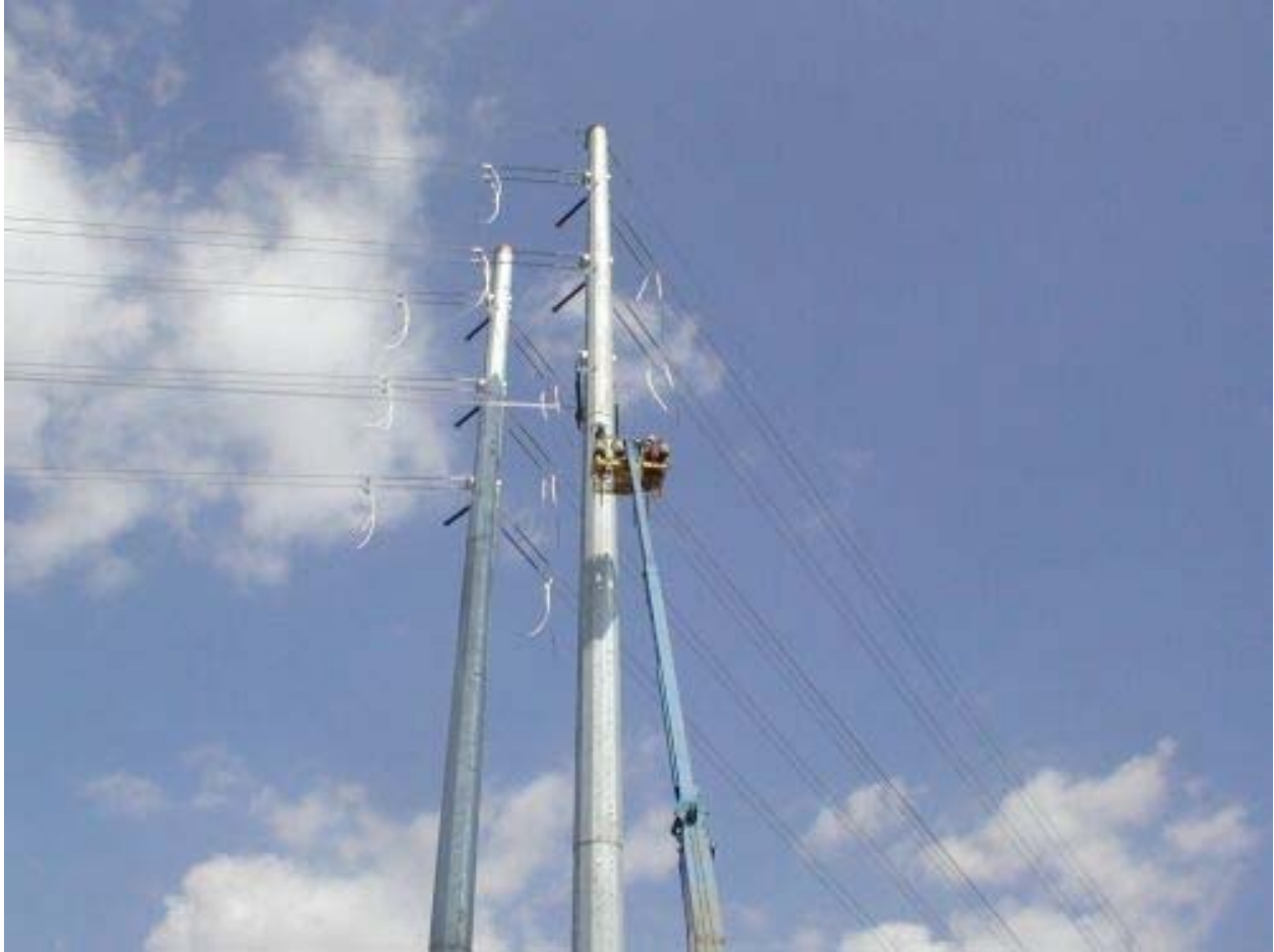
Figure 3 Crews Dead-ending Wire at Poles #14 L and R Along McCarthy Boulevard April 18, 2003
