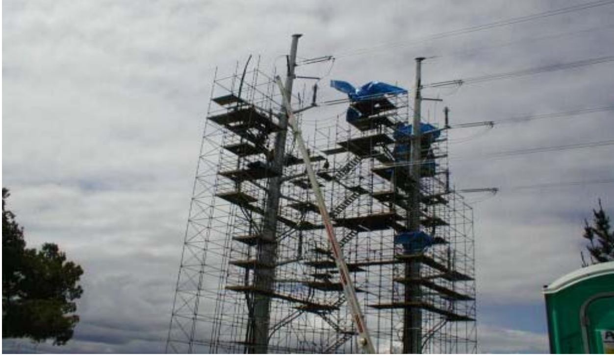
Figure 1 Scaffolding Around Poles #9 L and R at the West End of Cushing Parkway April 17, 2003
