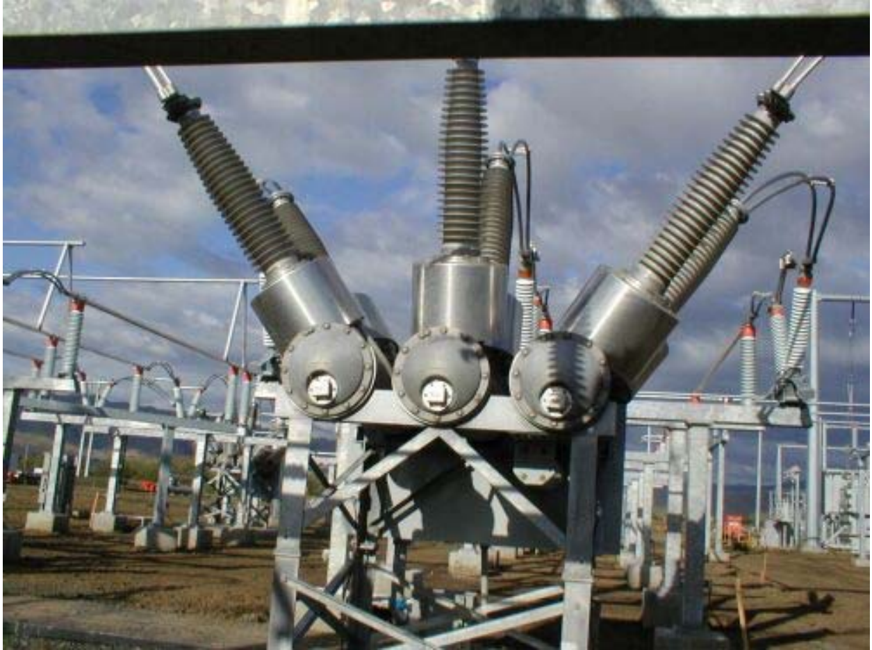
Figure 1 House Finch Nesting in Insulator Structure at Los Esteros Substation (small square box in left circle) April 24, 2003
