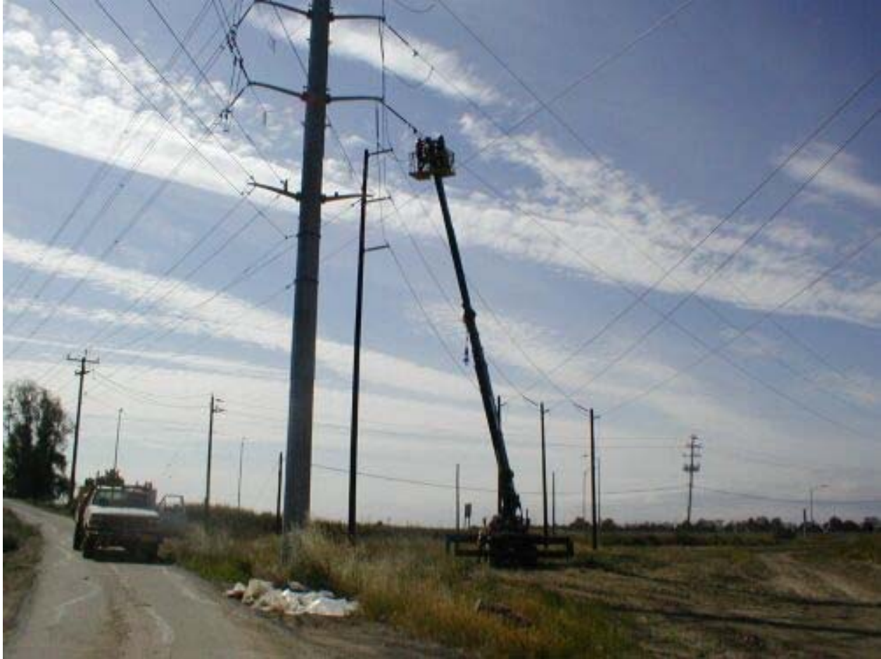
Figure 1 ILB Crews Working at Pole #30 in the Field West of the Los Esteros Substation May 24, 2003
