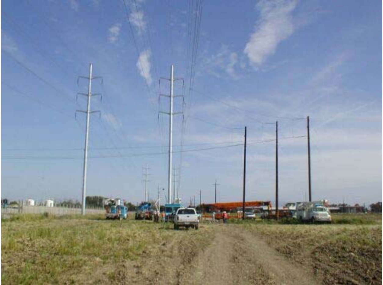
Figure 2 PG&E Crews Working in the Field West of the Los Esteros Substation May 24, 2003
