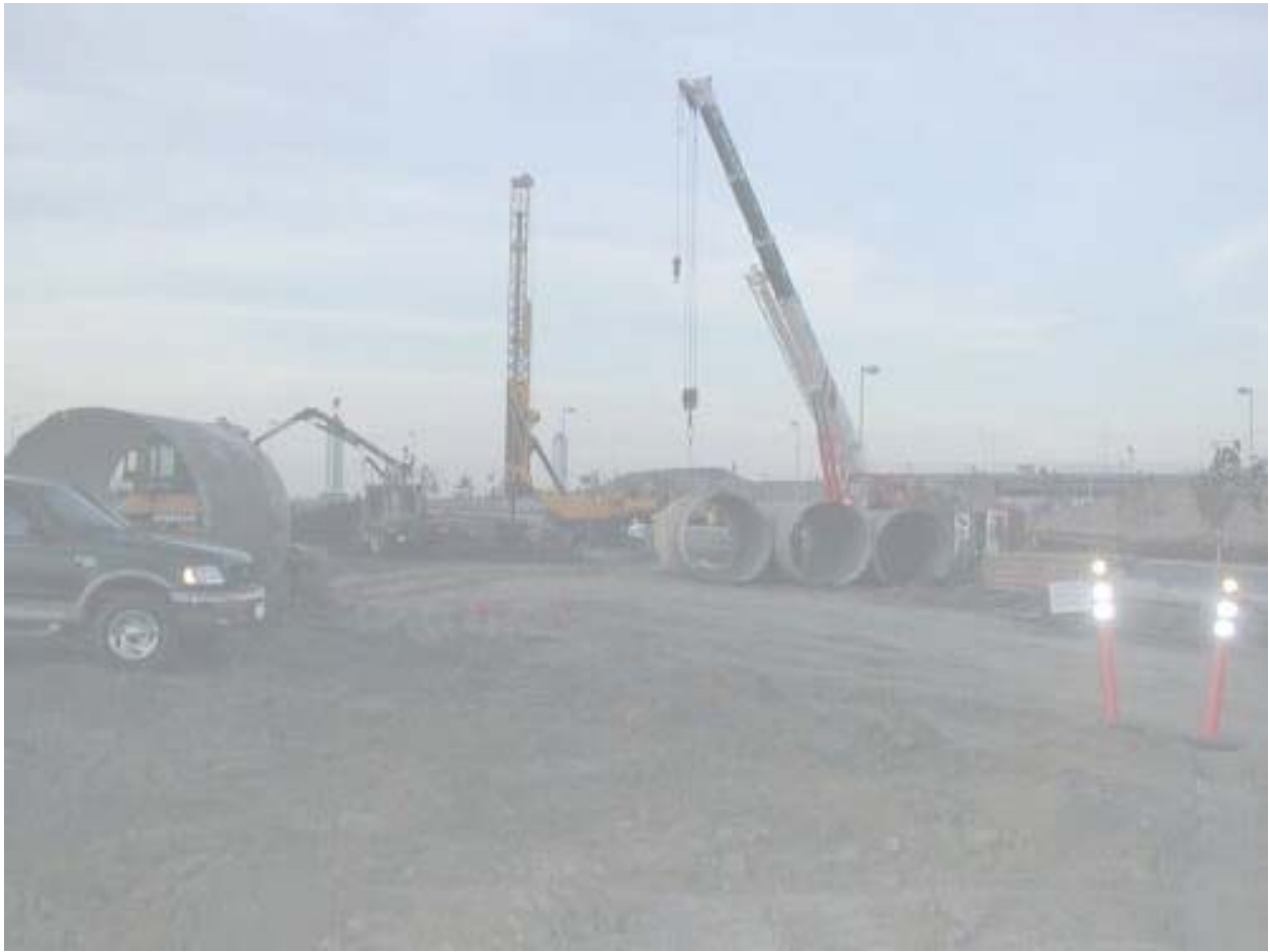
Figure 3 Foundation Work for Poles #15 (a) and (b) of the Overhead Segment November 20, 2002
