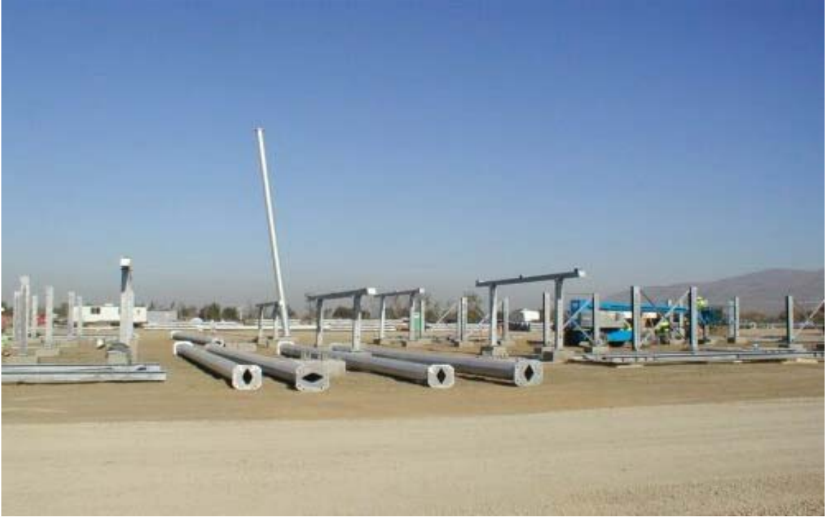
Figure 2 Los Esteros Substation: Steel Pole Structures November 27, 2002
