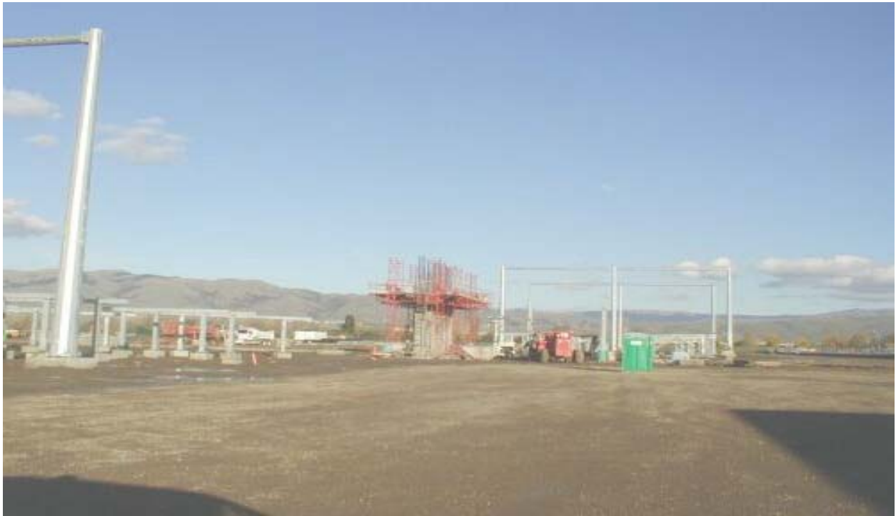
Figure 6 Wall Being Built at the Los Esteros Substation Site (with red scaffolding around it) December 18, 2002
