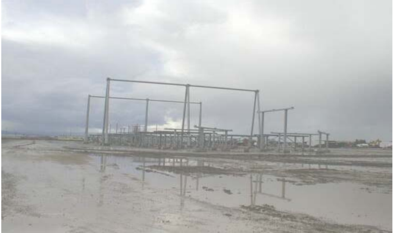
Figure 3 Los Esteros Substation After Big Storm Event December 17, 2002
