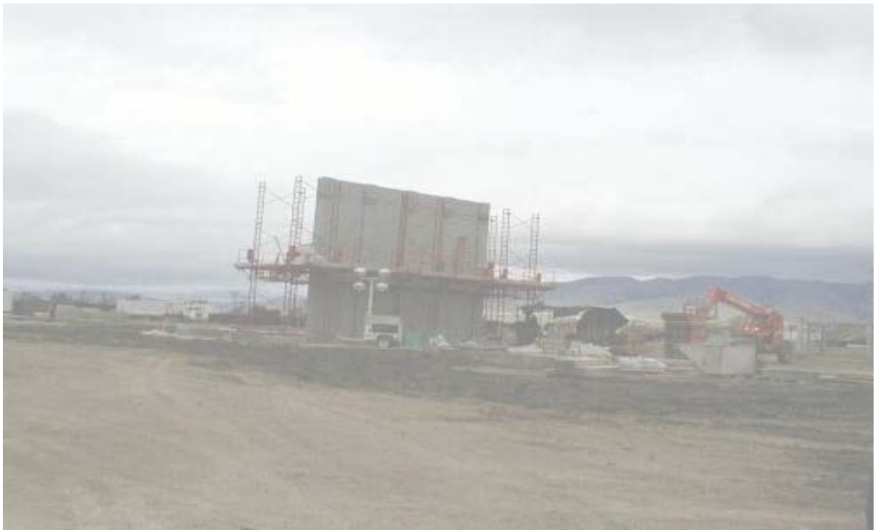
Figure 4 Crews Building a Fire Wall at the Los Esteros Substation Site December 27, 2002
