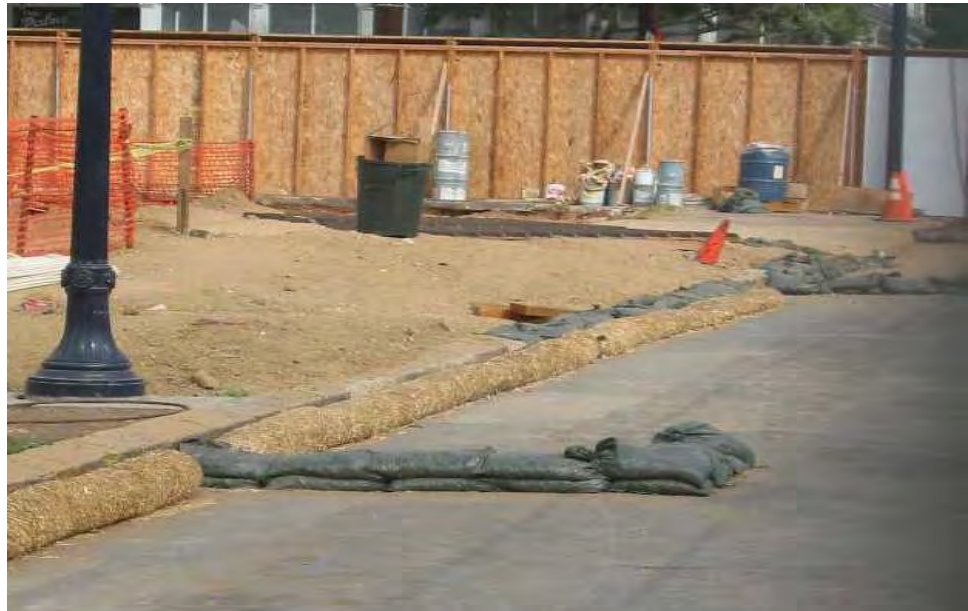
Gravel bags and fiber rolls used as a perimeter sediment control system.
