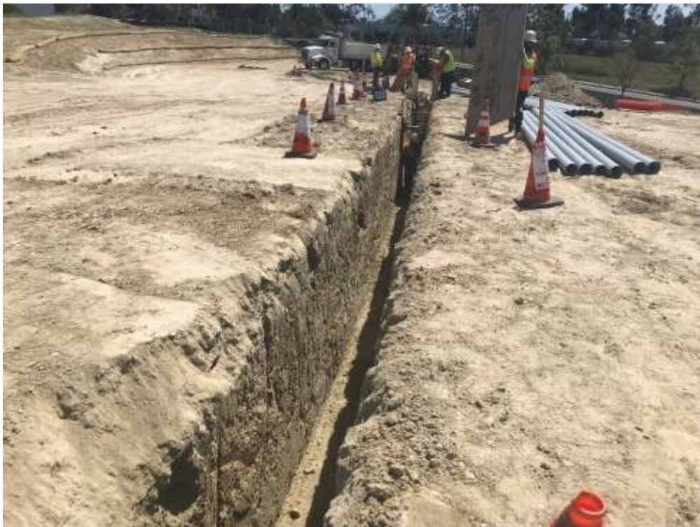
Figure 2 – Excavation of the trench followed by conduit installation for the on-site distribution system.
