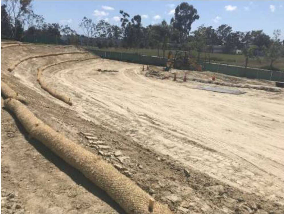
Figure 1 – The new driveway from Avenida Del Oro was graded and BMPs were installed.
