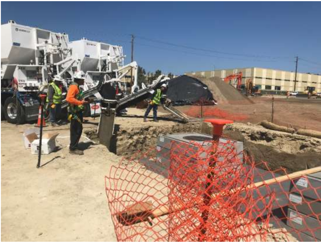
Figure 3 – Vaults for the on-site distribution system were set then were backfilled with slurry.
