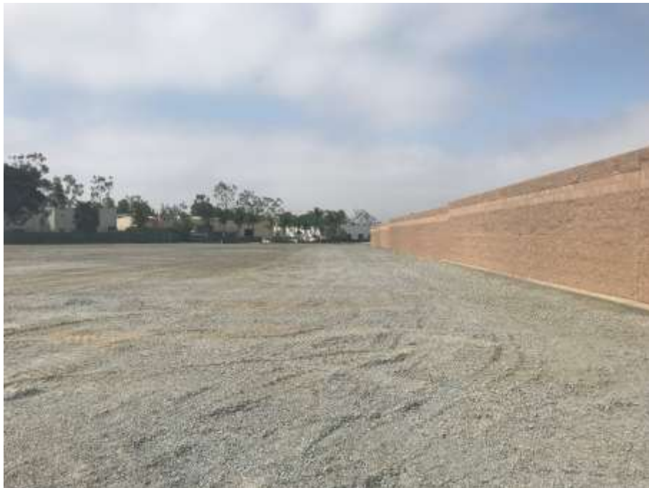
Figure 2 – Class 2 base rock and perimeter block wall was installed around the future substation site, July 25, 2018.
