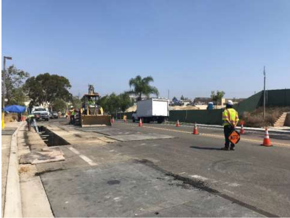
Figure 3 – Trenching and conduit installation for the Loop in work being conducted along Avenida Del Oro, July 25, 2018.
