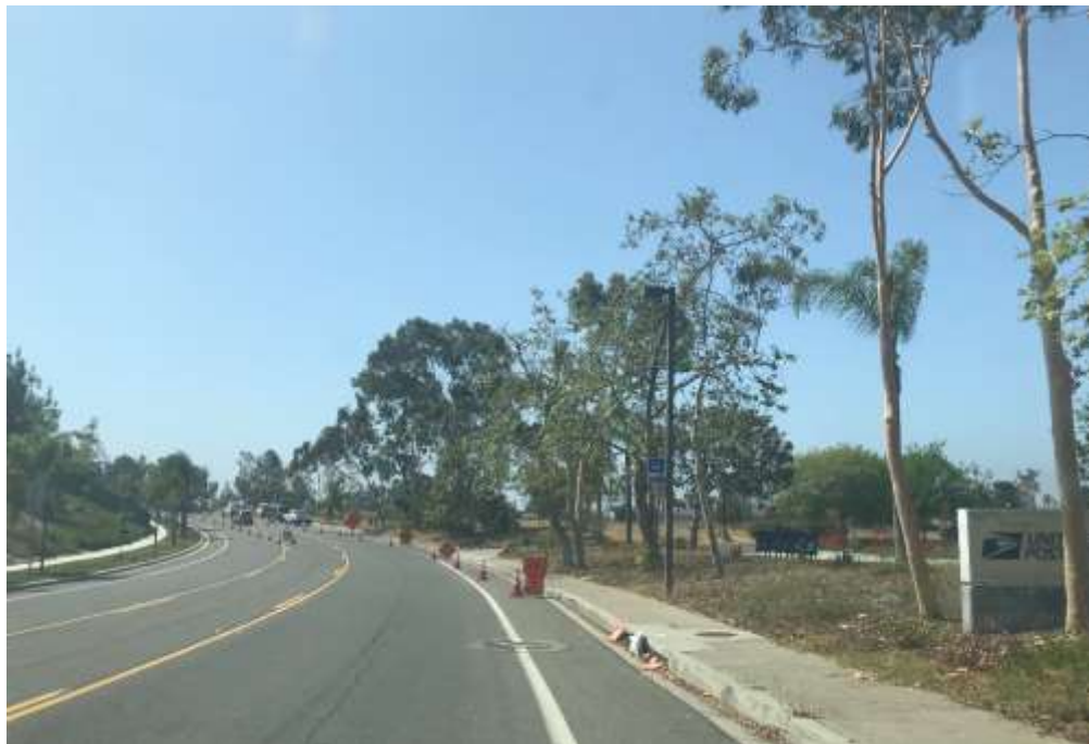
Figure 4 – Traffic controls are in place and lanes are open during construction on Avenida Del Oro, July 25, 2018.
