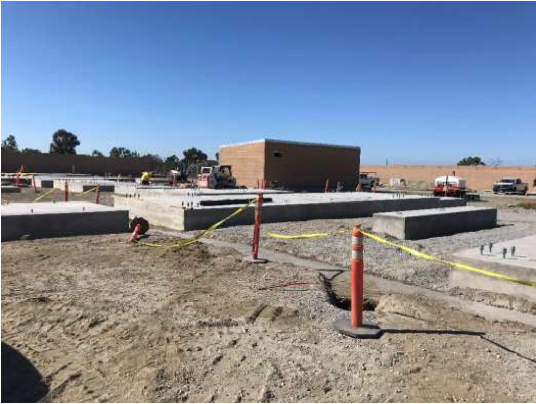
Figure 1 – Foundation construction and control shelter construction continue at the Ocean Ranch Substation, October 31, 2018.
