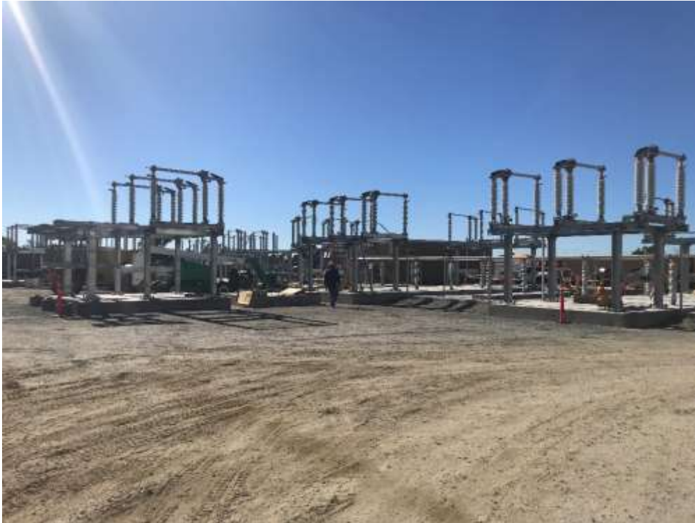
Figure 1 – Steel and insulator installation on foundations at the Ocean Ranch Substation, January 23, 2019.
