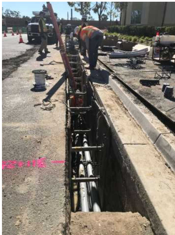
Figure 4 – Trenching on Rocky Point Drive was followed by conduit installation and concrete backfill, January 23, 2019.
