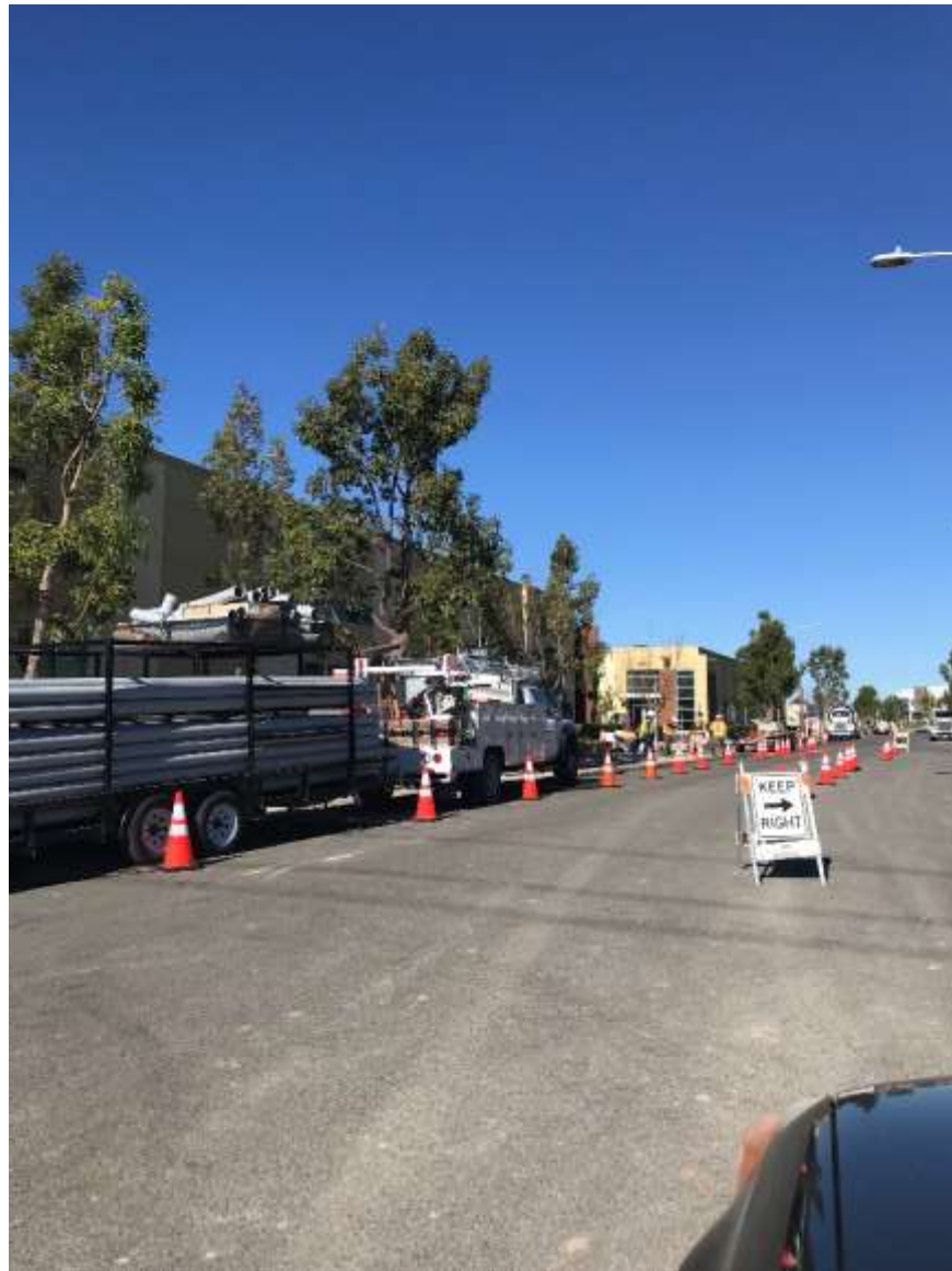
Figure 5 – Traffic control set up for the 12-kV underground work along Rocky Point Drive, January 23, 2019.
