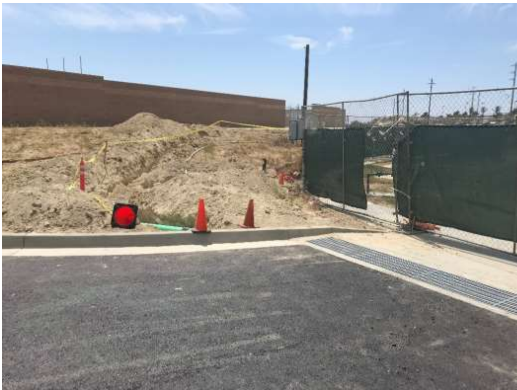
Figure 4 – Main line irrigation installation for landscaping of the areas outside of the Ocean Ranch Substation, July 23, 2019.
