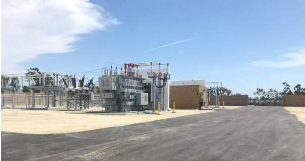
Figure 1 – Crews completed final paving of the interior access road within the Ocean Ranch Substation, July 23, 2019.
