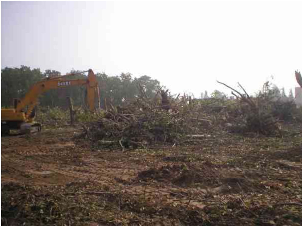
Figure 4 – Wood debris piles, November 1, 2007.
