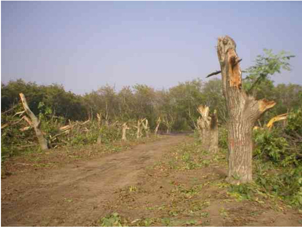
Figure 1 – All of the walnut trees at the future substation site have been topped off, November 1, 2007.
