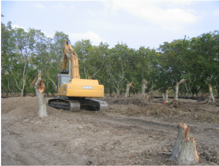
Figure 1 – An exactor is used to remove the tree stumps and roots from the new substation site, November 9, 2007.
