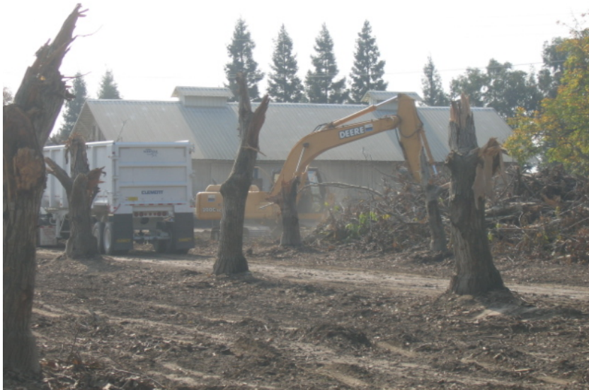
Figure 2 – A second excavator loading the tree stump debris into trucks for chipping off site, November 9, 2007.
