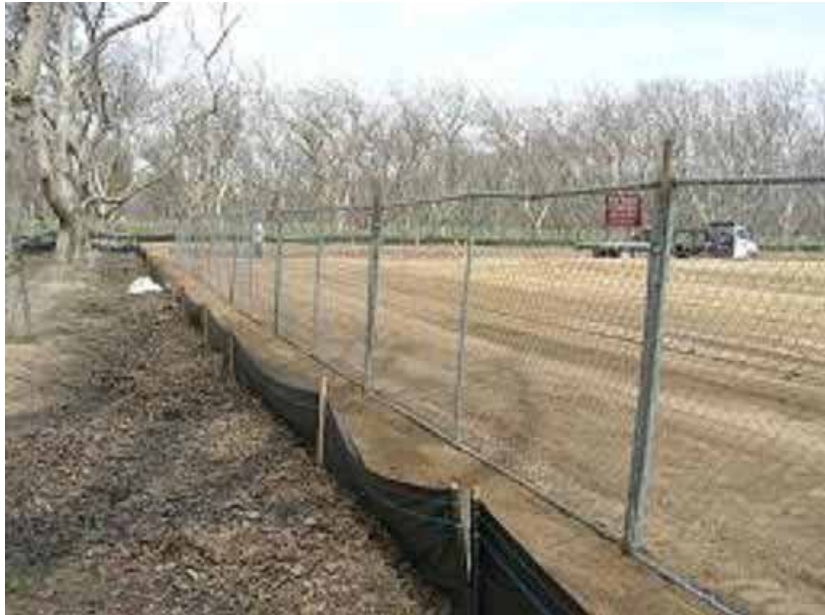
Figure 4: Silt fencing had been installed around the entire substation boundary before any construction activity occurred. The perimeter chain link fence was installed by the civil contractor.
