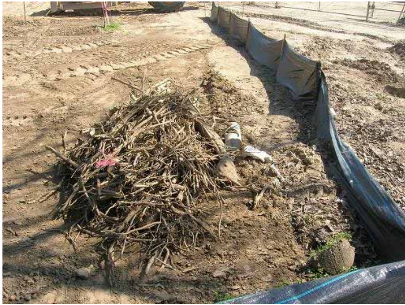
Figure 3: During the excavation processes, the walnut tree roots remaining from the tree removal stage of the Project were gathered and removed from the site.
