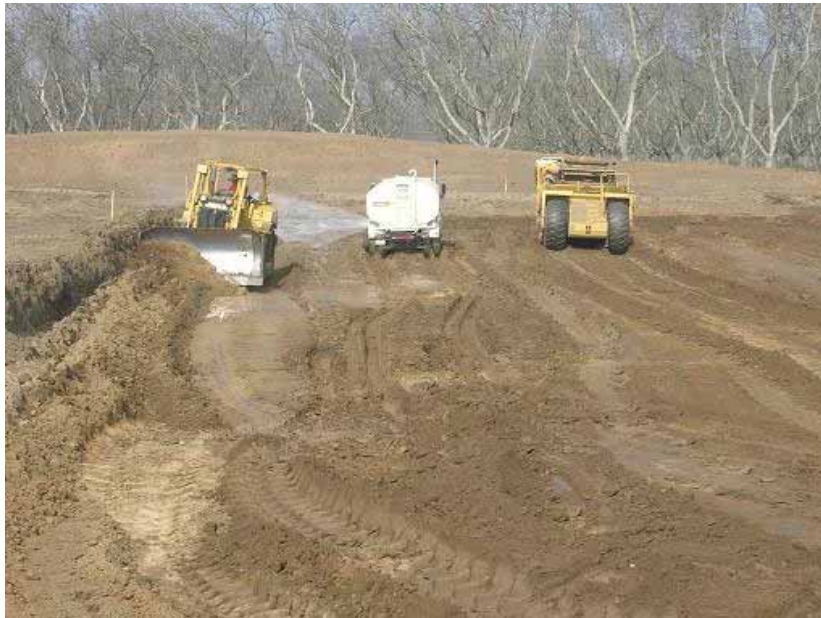
Figure 2: Site grading involved excavating material, moving it, storing it within the site, and then repositioning it using water and mechanical means to achieve required compaction and moisture content.
