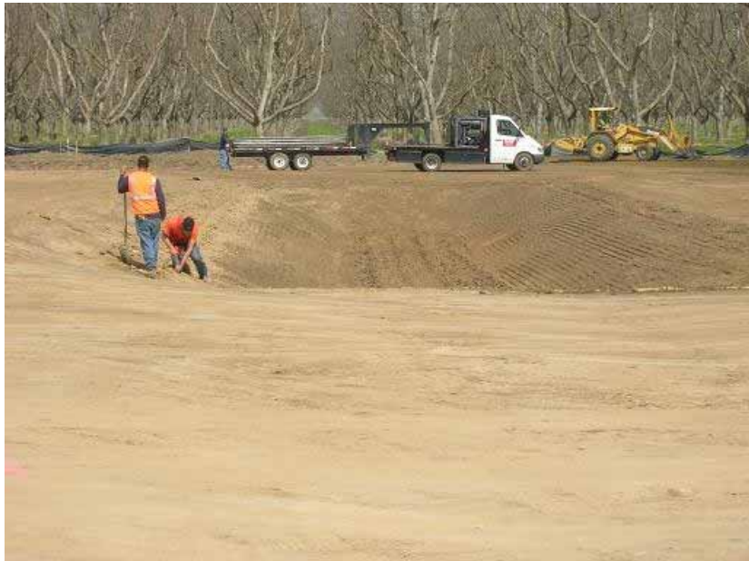
Figure 5: The civil contractor began construction activities with the excavation of the retention basin.
