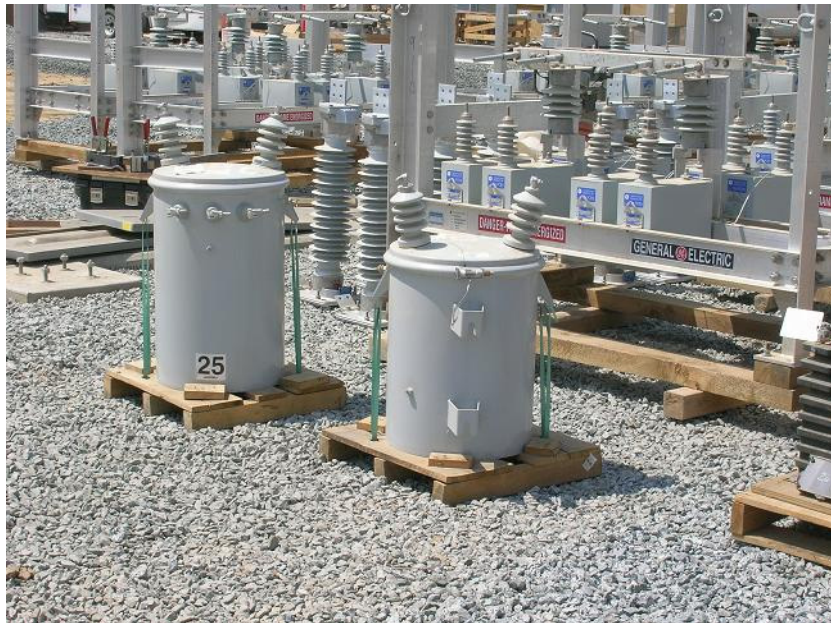
Figure 4: Capacitors also have been hauled to the site and were in the process of being installed.
