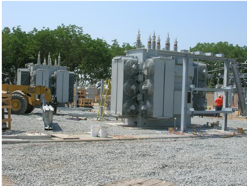
Figure 3: The transformers have been hauled to the site and were in the process of being installed. The photograph faces northwestward.
