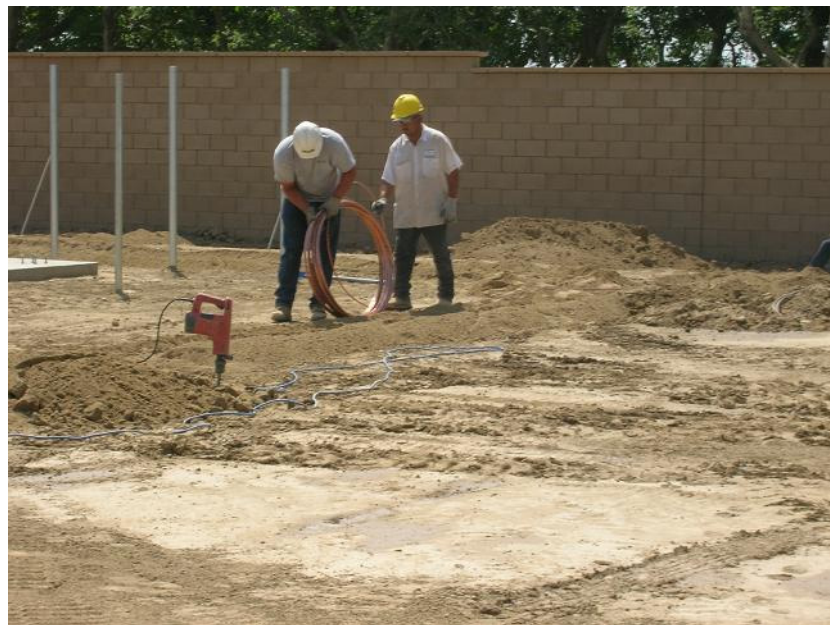
Figure 2: Installation of electrical conduit was another civil construction activity still underway. The adjacent walnut grove is visible behind the north perimeter wall.
