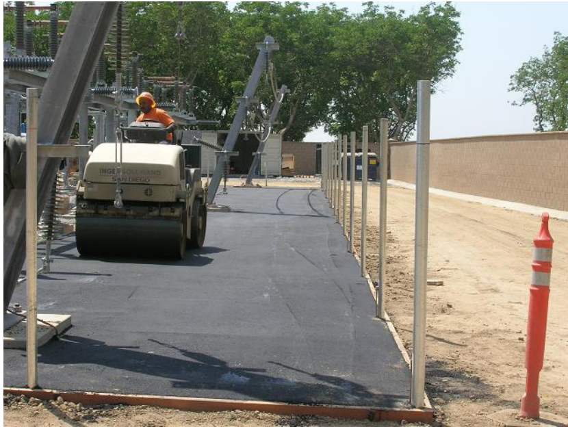
Figure 1: One of the last of the civil construction activities at the site was the placement of asphalt pads. The photograph faces westward. The north perimeter wall is on the right.
