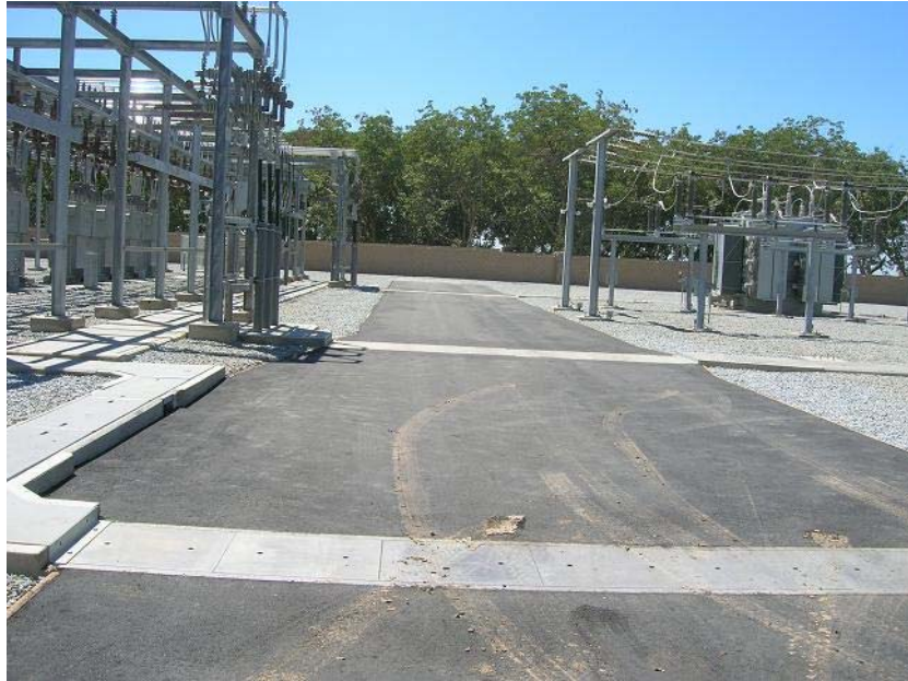
Figure 1: The two paved roadways within the substation have been completed. The photograph faces westward.
