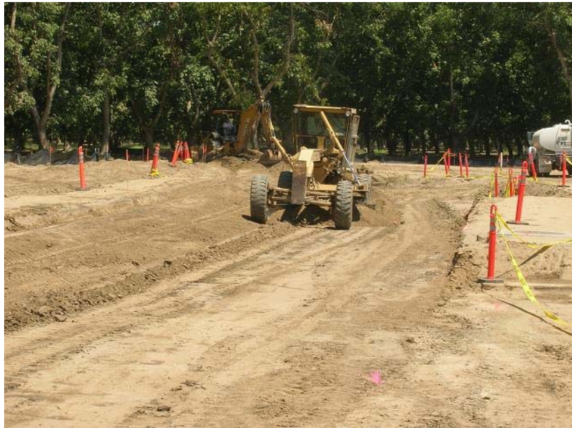
Figure 2: The landscaping contractor has begun construction of the road outside the north border of the substation. The photograph faces eastward.
