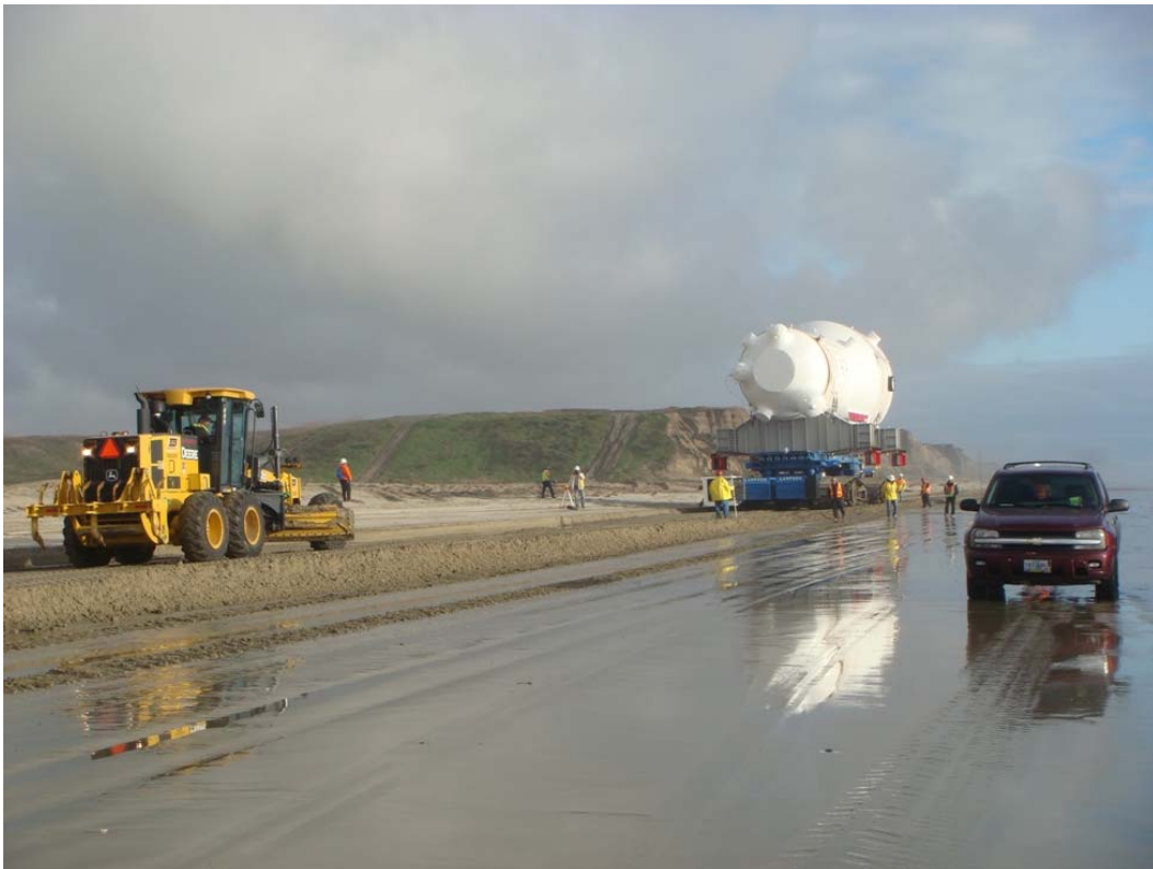
Figure 2: The beach route was prepared using graders and bulldozers below the mean high tide line to create an even driving surface for the crawler.
