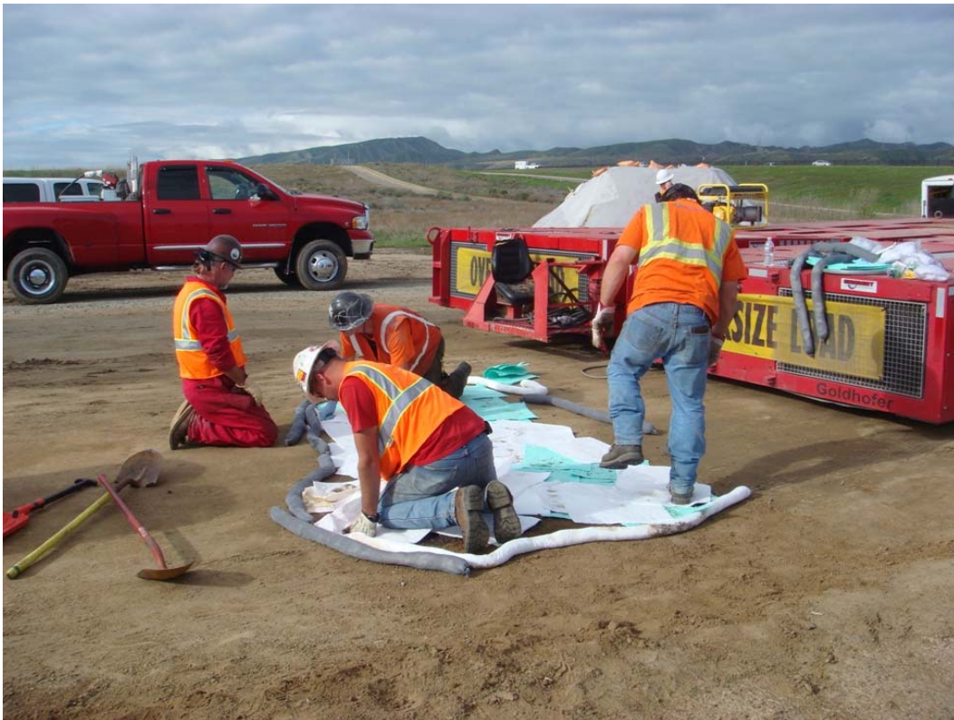
Figure 6: SCE Haz Mat crews responded to a hydraulic spill from the Goldhofer at the Las Pulgas staging area.
