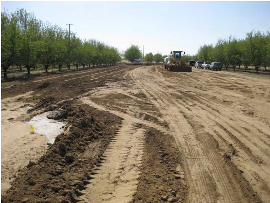
Figure 2: The access will be paved. At present a shaker plate and rock apron are located at the entrance to Seventh Standard road behind the photograph, which faces southward.
