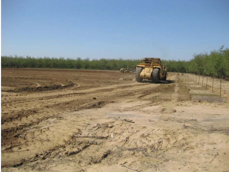
Figure 1: Grading of the site began during the week of March 8, 2010. The site has been demarcated by fencing. The photograph faces westward.
