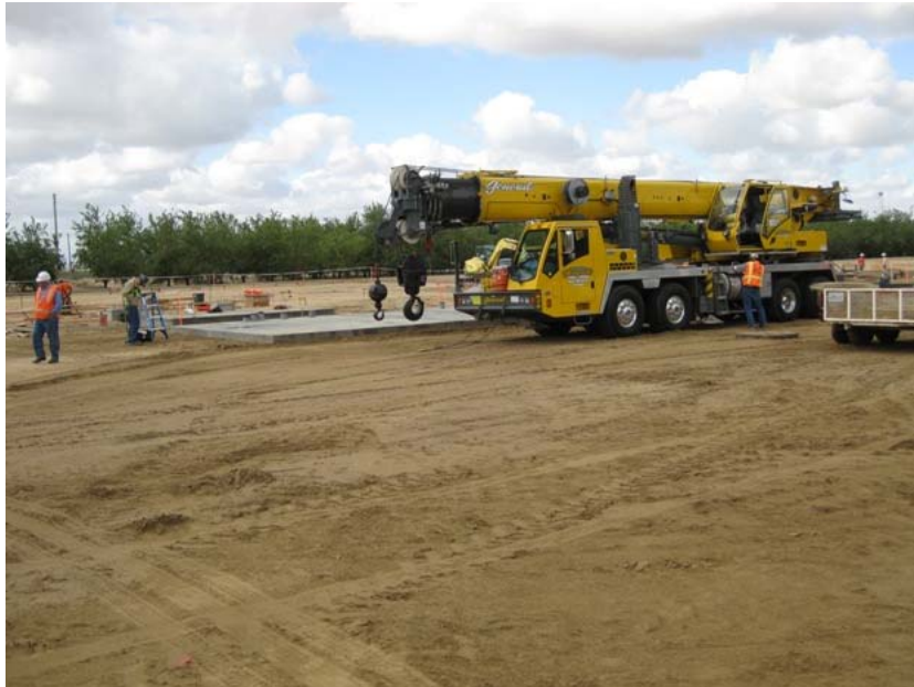
Figure 3: The controls enclosure was erected and bolted on to its concrete pad during the last week of the subject period. The crane in front of the pad is positioned to receive the four sub-units of the enclosure that were brought on site by flat bed trucks. The enclosure pad is in the northeast corner of the substation site. The photograph faces southwestward.
