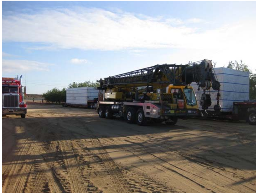
Figure 1: Equipment and materials for the installation of the electrical controls enclosure (Modular Protection Automation and Control enclosure) were hauled to the site immediately after NTP #2 was issued. The photograph was taken in the access road and faces northward.
