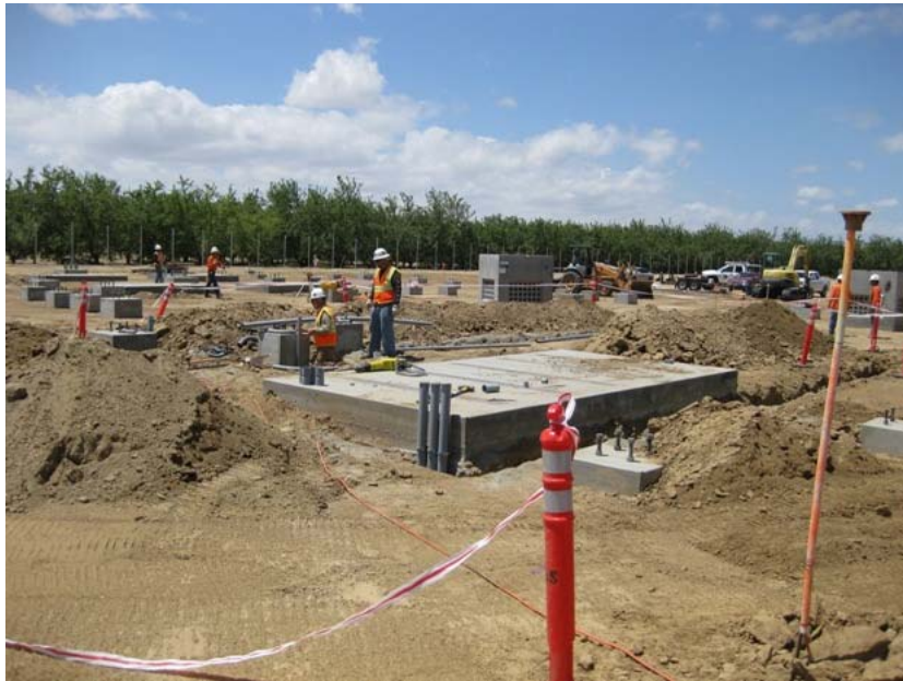
Figure 2: Construction of structure foundations and below-ground conduit trenches continued during the subject period. The photograph faces southwestward.
