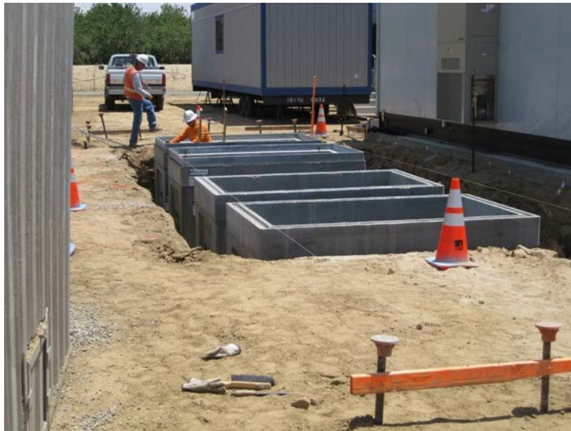
Figure 3: Vaults for the incoming electric lines have been placed next to the electrical control enclosure (to the right). One of the construction office trailers is in the distance. The photograph faces eastward.
