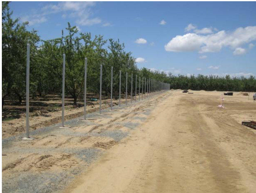
Figure 5: Poles for the perimeter chain link fencing were being installed during the subject period. The base rock that will cover the substation pad has been laid in the path of the fencing prior to its installation. The photograph shows the south perimeter section, and faces westward.
