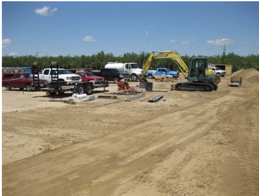
Figure 7: The western portion of the site will not be used for the current substation. It may be used for future substation expansion. During construction it is being utilized for vehicle and equipment parking, and for materials storage. The Biological Monitor and inspectors check this area several times each day for leaks, trash, open pipes, animals under equipment, etc. The photograph faces northwestward.
