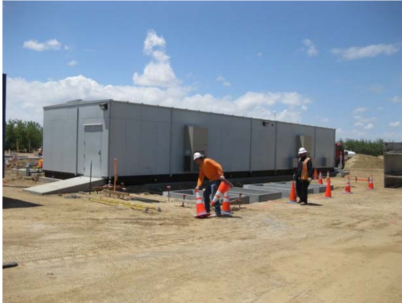
Figure 1: The electrical controls enclosure has been installed. It was hauled on site in four sections, and then assembled and bolted to its concrete pad. The photograph faces southwestward.
