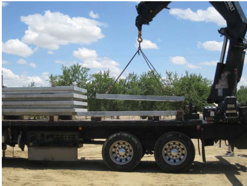
Figure 4: Lids for the incoming electric lines vault were installed during the subject period. The photograph faces eastward.
