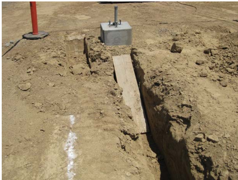
Figure 8: Construction involves the temporary excavation of many trenches and holes for foundations and conduits. All holes are covered overnight, and deep trenches are provided with ramps. These features are regularly checked by the biological monitor.
