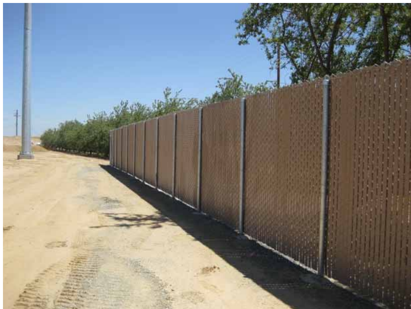
Figure 4: Construction of the perimeter chain-link fence continued during the subject period. The photograph faces northward toward the access road and Seventh Standard Road. One of the three recently installed tubular towers stands in the middle distance.
