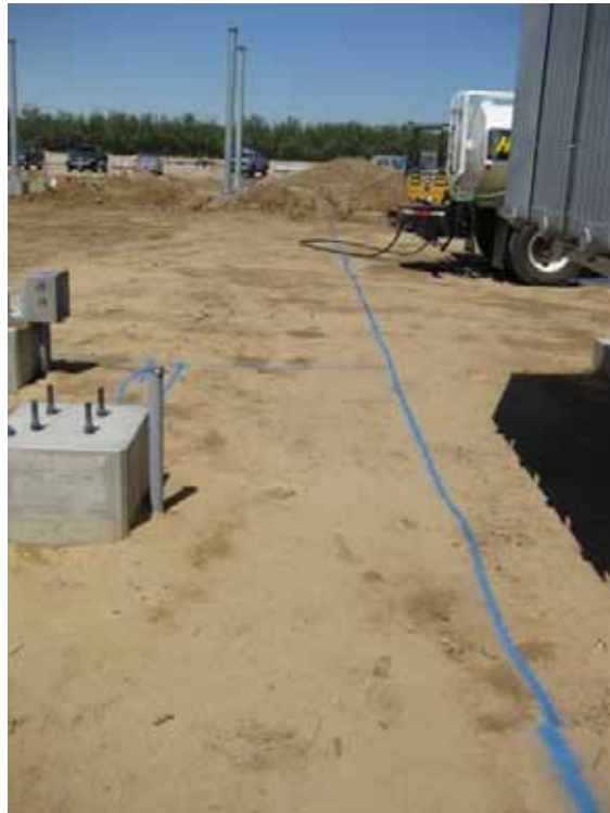
Figure 2: During the subject period, installation of the ground grid system continued. Narrow trenches were excavated along the blue lines. If left open overnight, they were checked by the biological monitor for animals before commencement of work in the morning. The photograph faces westward.
