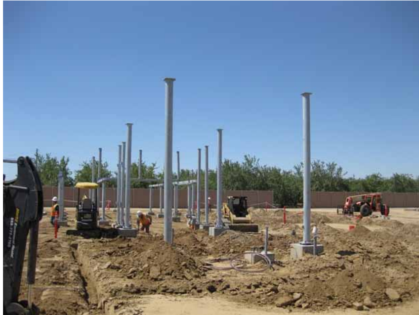
Figure 1: During the subject period, erection of structures began. Construction of below-ground conduit trenches and the ground grid system continued. The photograph faces southward.
