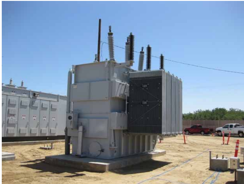
Figure 3: The transformer was hauled onsite and installed on the previously poured pad. The electrical controls enclosure is behind the transformer on the left. The photograph faces northeastward.
