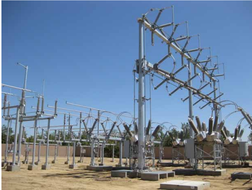
Figure 1: Erection of structures continued during the subject period. The photograph faces southeastward.
