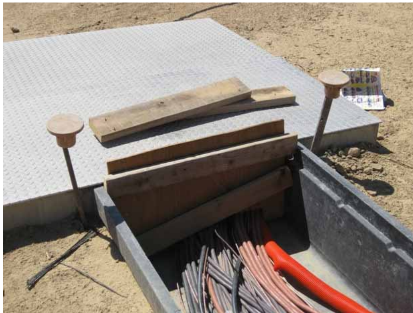
Figure 2: Construction of below-ground conduit trenches and installation of wiring continued. An opening from a conduit trench into a closed underground vault was blocked (wood covering in shaded area) to prevent usage by foxes and other animals.
