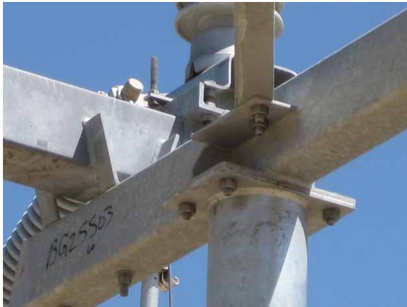
Figure 3: Several Project structures and construction facilities create potential nesting opportunities for several bird species. This small shaded ledge on the partially completed substation structure is an example. The measures put in place to discourage nesting by bird species have been successful to date.
