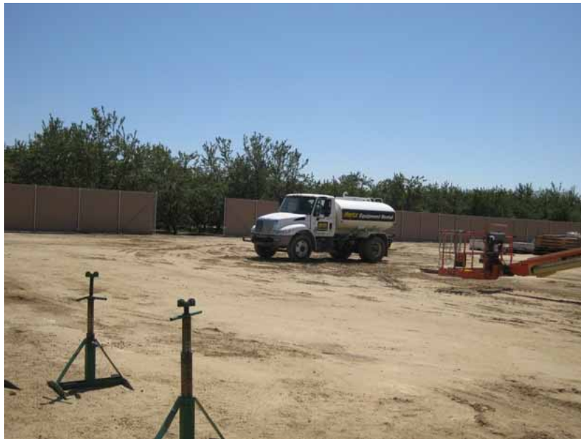
Figure 4: The contractor continued to use water trucks for dust control. Especially important has been the preparation of the soil surface at the end of each work week in order to prevent fugitive dust from occurring during the weekend. The photograph faces southwestward.
