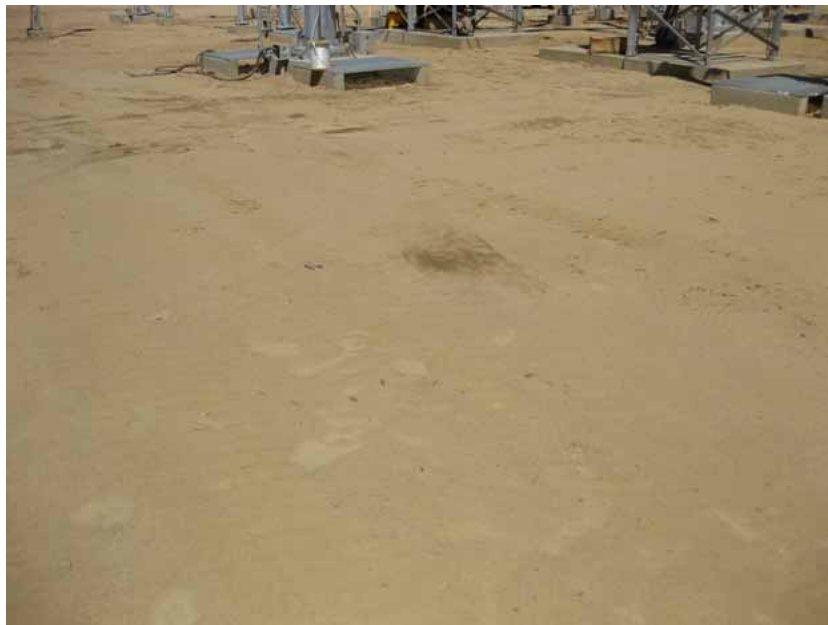
Figure 4: Water trucks continued to be used for dust control. Watering occurred on dirt surfaces on the entire site as much as three times per day when necessary. At the end of each work day, the site surface consisted of either well-compacted dirt, or, in areas recently disturbed, the loosened soil had a fairly thick crust from watering.
