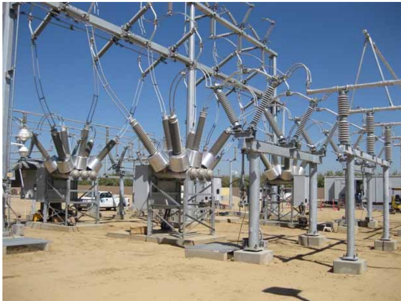
Figure 2: The primary electrical contractor, TTR, continued erection of structures. The photograph faces southwestward.
