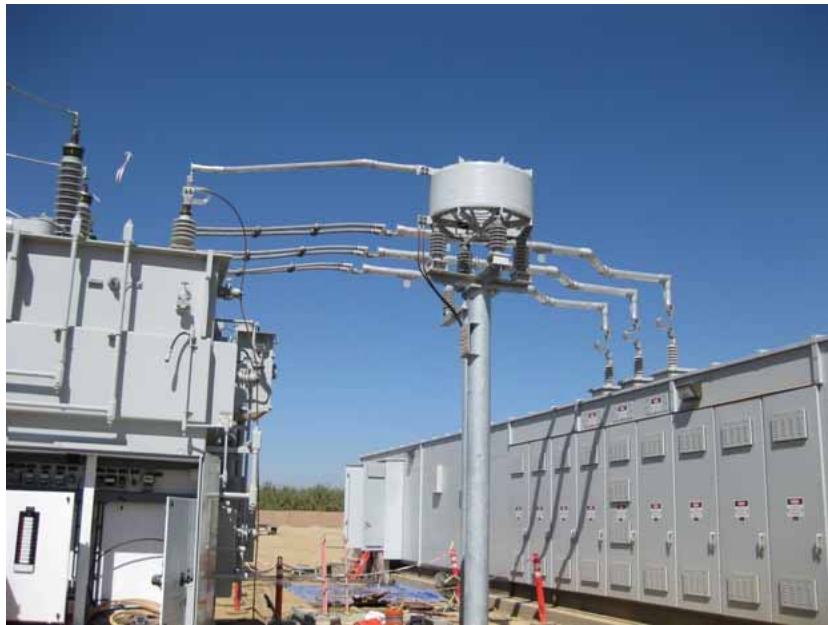
Figure 3: Connections between the structures housing the buses (to the left of the photograph), the transformer (on the left), and the electrical controls enclosure (on the right) were mostly completed during the subject period. The nine panels that will receive wiring from the transformer can be seen on the side of the enclosure. The photograph faces westward.
