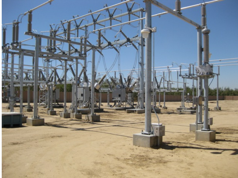
Figure 1: During the subject period, erection of structures was completed. Connections between the structures housing the buses, the transformer, and the electrical controls enclosure were completed. The photograph faces southwestward.
