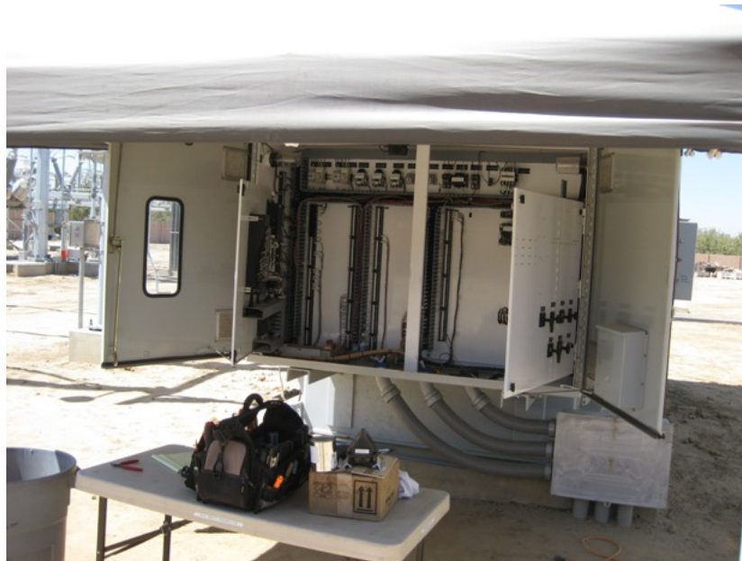
Figure 2: Detailed electrical installation and testing continued during the subject period. The photograph was taken at the transformer, and faces southwestward.
